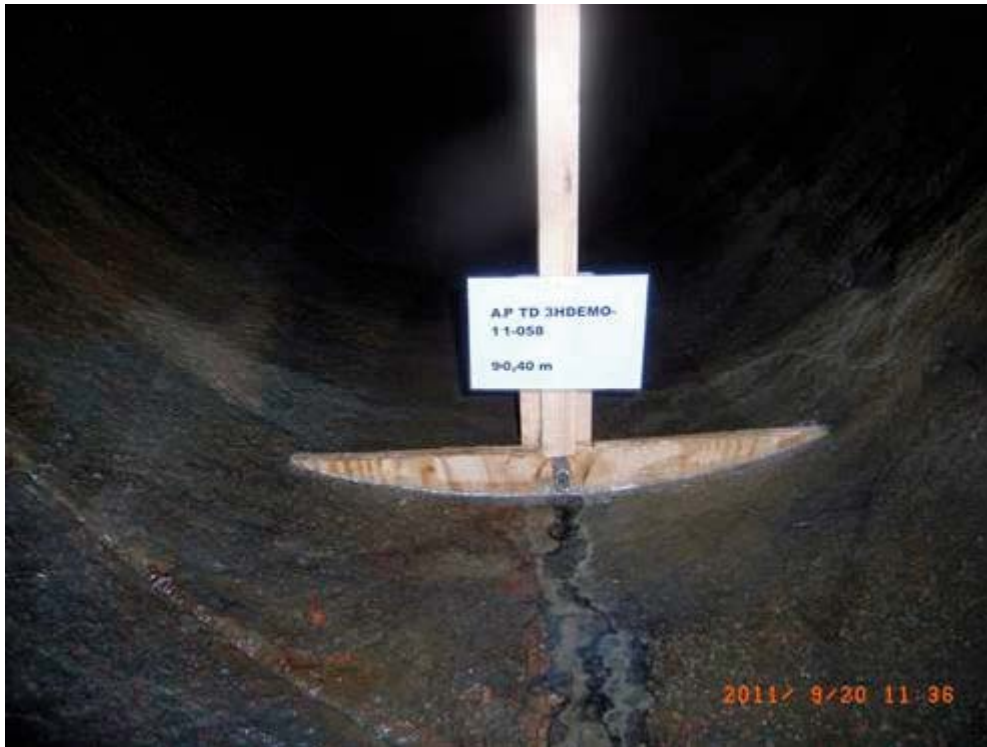
Figure 1-3. Wooden weir used to enable monitoring of groundwater inflow into the MPT drift.
