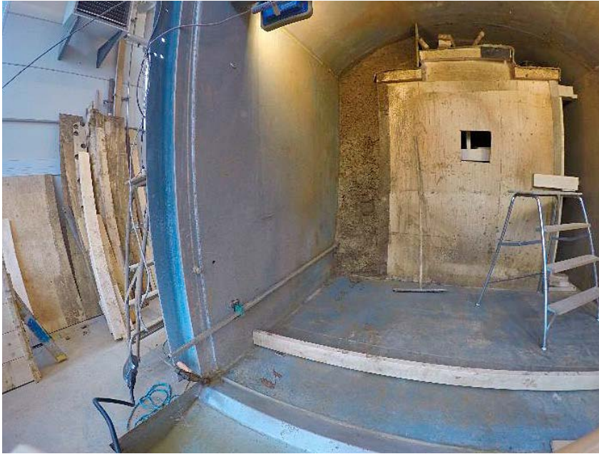
Figure 5-3. Photo showing the drainage pipe that was led out from the pellet filling.
