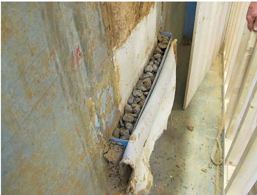
Figure 5-8. Photo showing the water collector. The geotextile has been removed from the top and the gravel filling inside the box can be seen. The photo was taken during excavation of the functional test.
