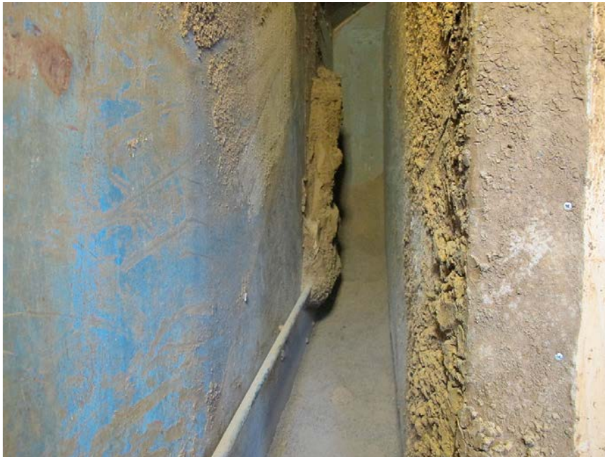
Figure 5-6. Photo showing the water collector during excavation. The box was covered with a wet layer of pellets.
