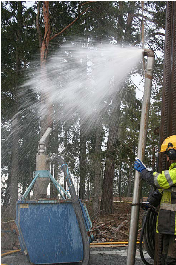
Figure 4-2. Cleaning of the telescopic section to 35.68 m of borehole KFM24 before the casing is installed. The air compressor supplies an ejector so that the mixture of water and drilling debris from the borehole bottom is flushed through the pipe up to the surface.
