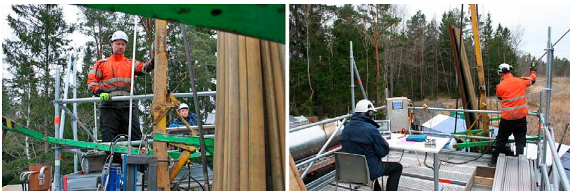
Figure 5-17. Left: The insertion rig engine was mounted in a firm foothold, and was centered and bolted on the beam 3 m up. Right: Measurement with the gyro. The instrument is attached to 20 mm steel rods, and the engine is set to move the probe one metre at a time when a measure is taken.
