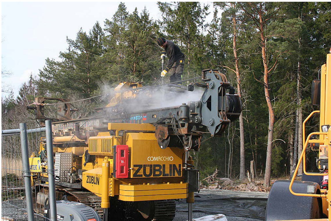
Figure 4-1. By using hot water the drilling rig and drill rods are washed before the equipment is moved into position on a concrete platform at the drill site.
