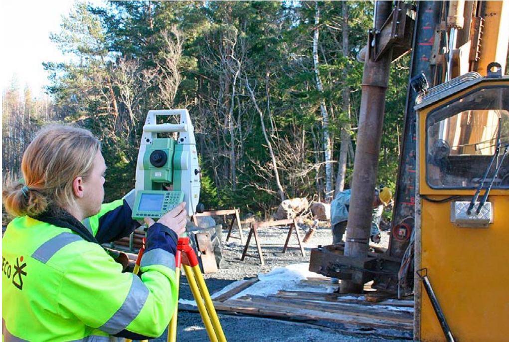
Figure 5-5. Reflectors are taped on the NO-X 280 casing, and with a total station measurement are performed so that the start direction can be calculated.
