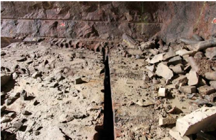
Figure 3-4. Completed slot next to the tunnel face. Parts of the slots were excavated by seam drilling, see upper part of the photo (Photo by Rickard Enér).
