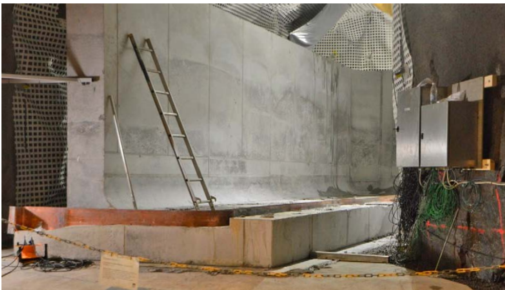
Figure 4-33. The concrete structure after dismantling of the formwork. The cabinet in the right part of the image contains equipment for data collection from the sensors in the concrete structure.
