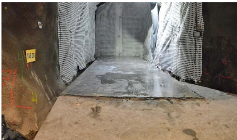
Figure 4-30. The tunnel (TAS 05) which was used for the test casting. In this image the tunnel has been prepared for test casting with a concrete base slab and means to secure the tunnel walls against rock fall-outs. The dimensions of the concrete base slab are 15 \times 4 meters and the available tunnel height is about 4.5 meters.
