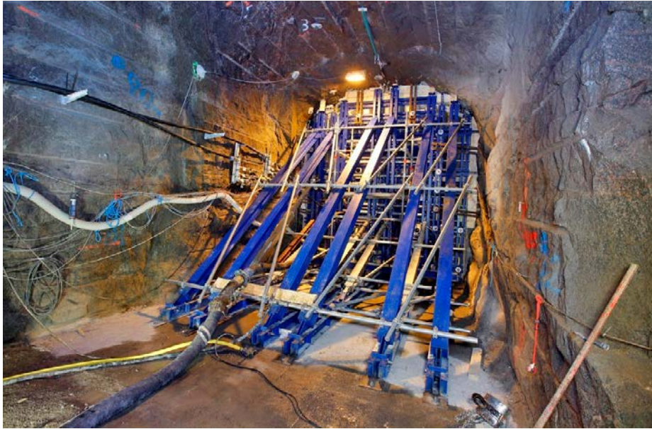
Figure 4-24. Concrete is pumped in behind the formwork for casting of the concrete dome structure.
