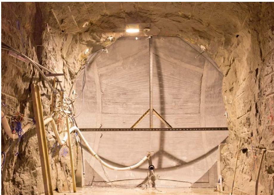
Figure 4-25. The hardened concrete dome structure after removal of formwork. The steel beams in front of the dome are used for displacement sensors.
