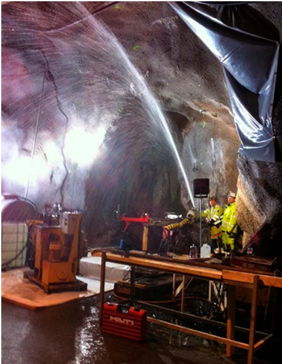
Figure 5-5. Grouting of K03009F01. To be able to insert the grouting packer by hand into the borehole at the length of 4.5 m, the valve must be open. When the packer is expanded, the groundwater inflow of 250 L/min with c. 30 bars overpressure creates an impressive outflow through the valve.
