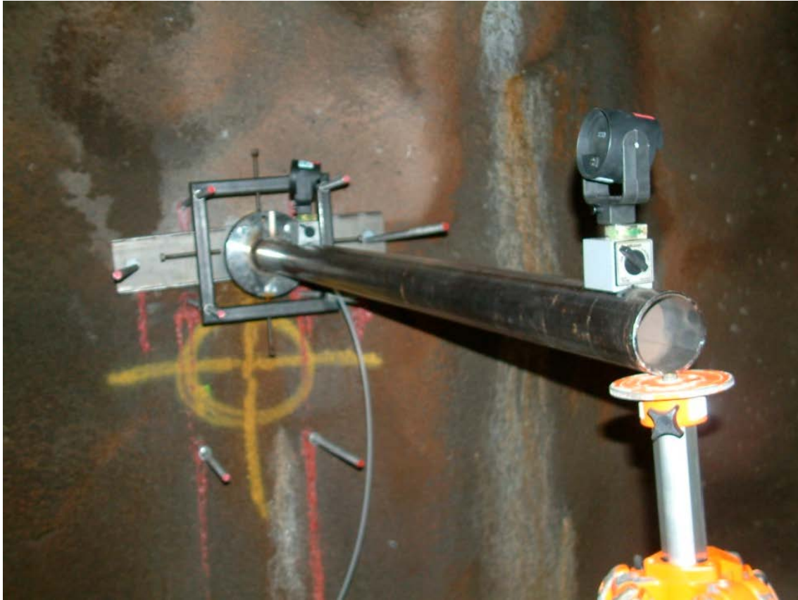
Figure 7-6. The casing was positioned and aligned prior to grouting. The bolts previously used for the plate on the rock were now used for positioning.
