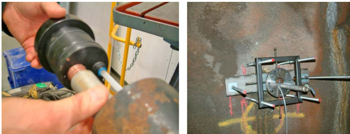
Figure 7-5. The casing was grouted from inside and out. Left: A plastic plug with lead-throughs for pumping in grout and evacuating the air was glued inside the casing. Standard cement was pumped through the aluminum tube and the plug and then filled the annular gap between the casing and the borehole wall. Right: Air evacuation pipe 8 mm and a frame with adjustable bolts.
