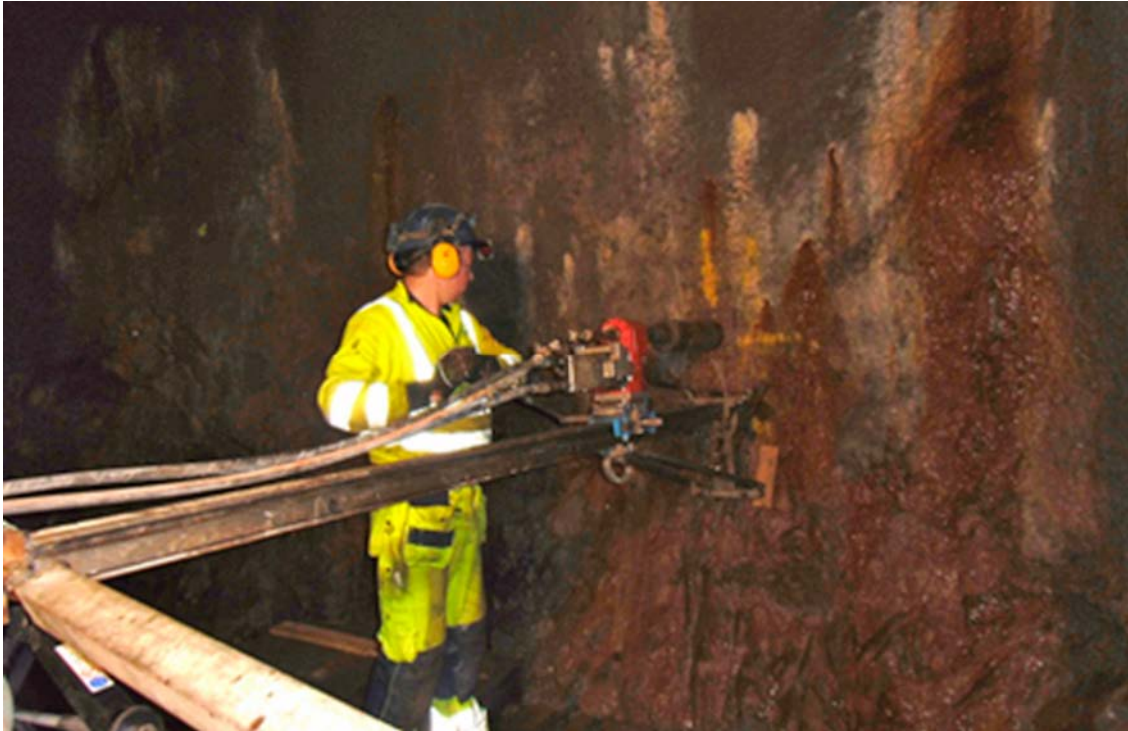
Figure 5-2. Pre-drilling of K03009F01 in TAS03. The tunnel wall is fractured and wet.
