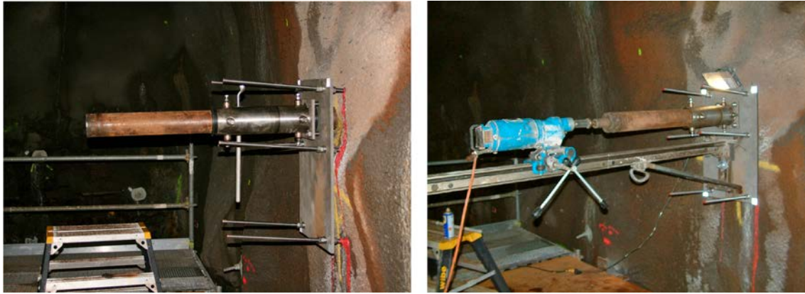
Figure 7-2. A steel plate was bolted to the tunnel wall perpendicular to the borehole axis. A steering tube adapted to the pre-drilling core barrel used was bolted on the steel plate and surveyed. The tight steering (small annular space between the steering tube and the core barrel), forced the core barrel to drill in the correct direction. A small drill rig was used for pre-drilling of the 2.28 m long casing borehole.
