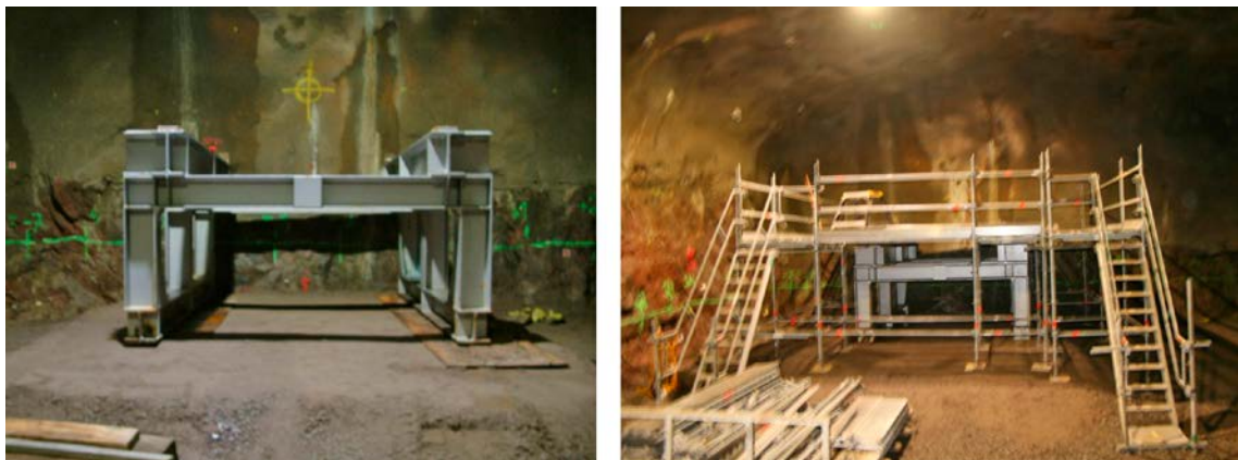
Figure 7-1. A solid fundament was placed on top of the aligned and hard-packed tunnel floor. A scaffold was built around the fundament, completed with safety equipment. Two separate staircases give access to the drilling rig from both sides of the scaffold.
