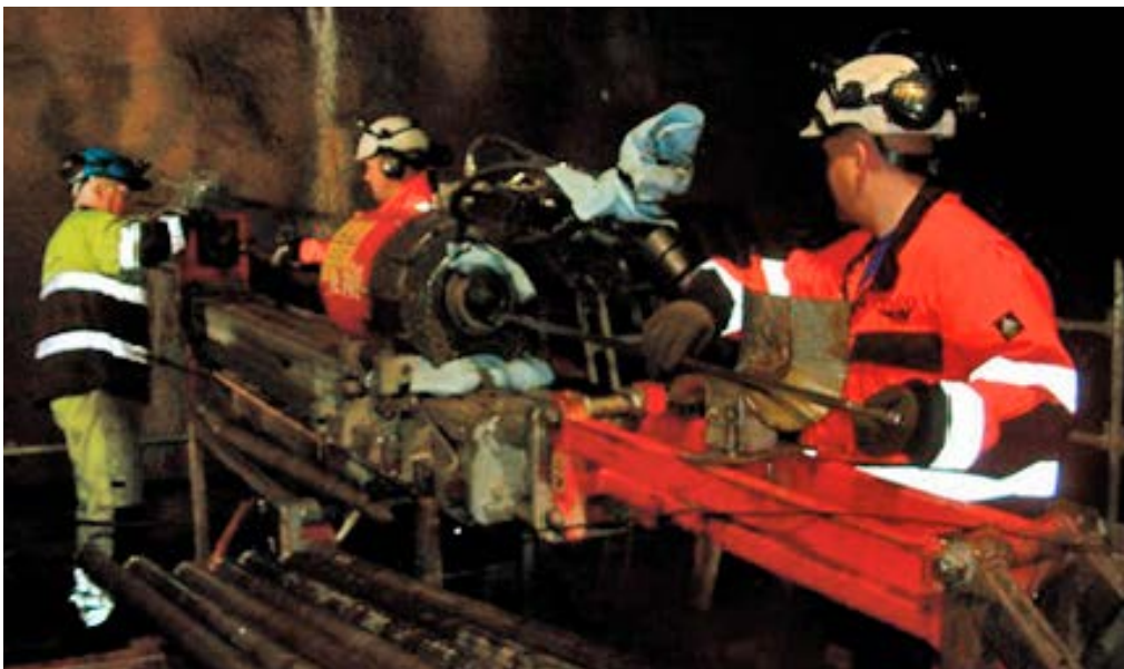
Figure 9-1. Technical problems with the hydraulic rotation unit initially caused a delay in the drilling process and also caused a minor oil leak, which had to be taken care of. Still, after exchanging the rotation unit, the drilling of K08028F01 could be completed on schedule.
