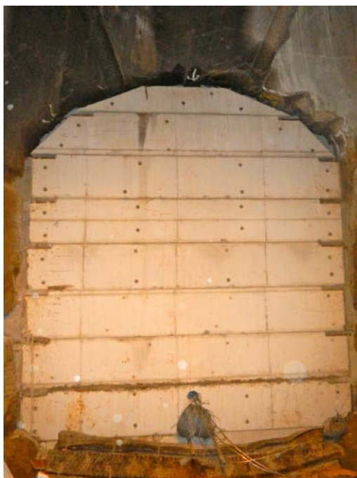
Figure 5-3. Photo taken during the installation of the plug test at Äspö. The photo shows the concrete beams outside the bentonite sealing (Sandén and Börgesson 2014).
