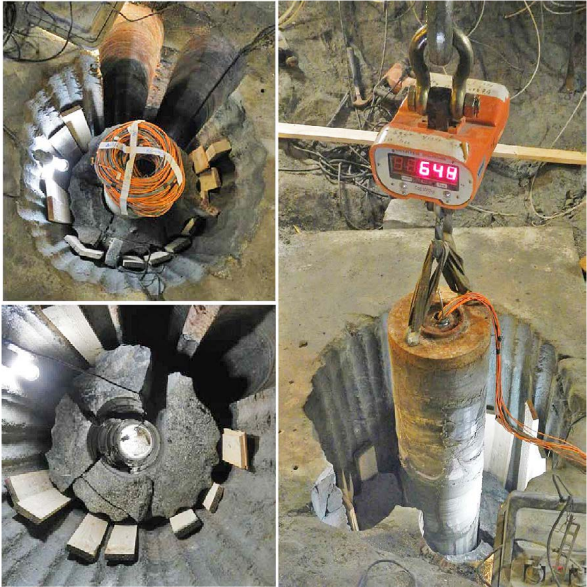
Figure 4-20. Pictures for dismantling of parcel in Hole 18. Wire-sawing completed (upper left), pulling of parcel (right), remaining rock blocks (bottom left)
