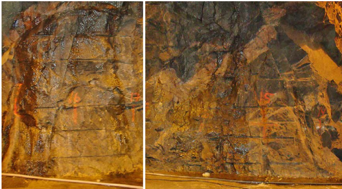
Figure 5-8. Photos of deformation zone in left and right wall. The deformation zone is complex and strike and dip was estimated based on structure 10 and 12 seen in Figure 3-25.
