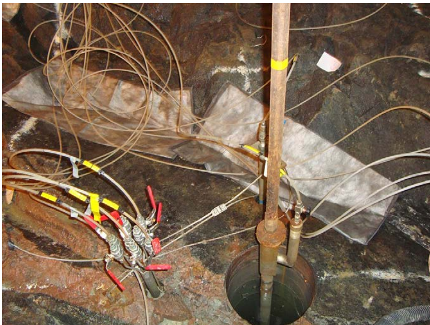
Figure 3-50. Sorbing mats used for tunnel flow measurements (mats 3-4 close to KO0018G01, see Figure 3-51). Mats located on the floor where wet spots were identified. Photo Åsa Fransson.
