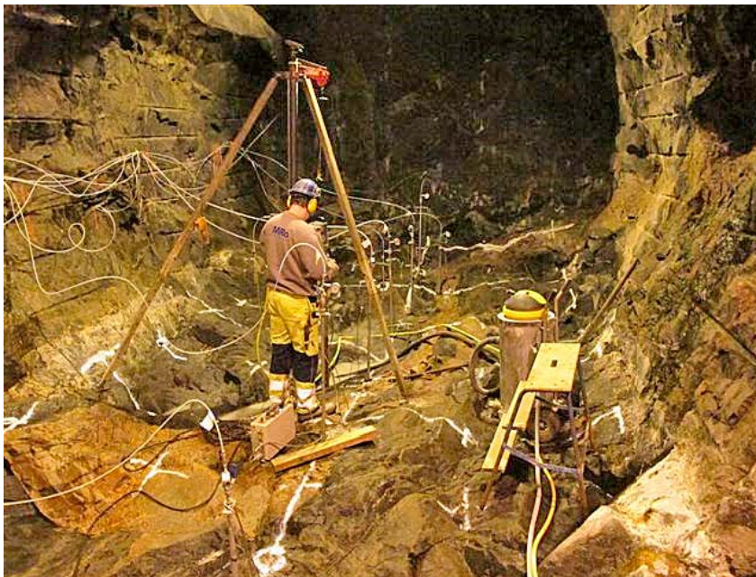
Figure 3-20. TASSO-tunnel (Phase 2) and the ongoing drilling of the additional 14 boreholes (tunnel floor), see geometry in Figure 3-1. The photo shows that the concrete slab has been removed.
