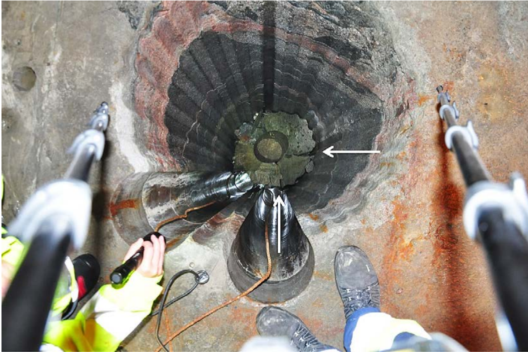
Figure 5-20. Borehole KO0017G01 following stitch drilling and dismantling. New (not previously identified) fractures being more or less parallel or perpendicular to tunnel and close to in line with adjacent boreholes.
