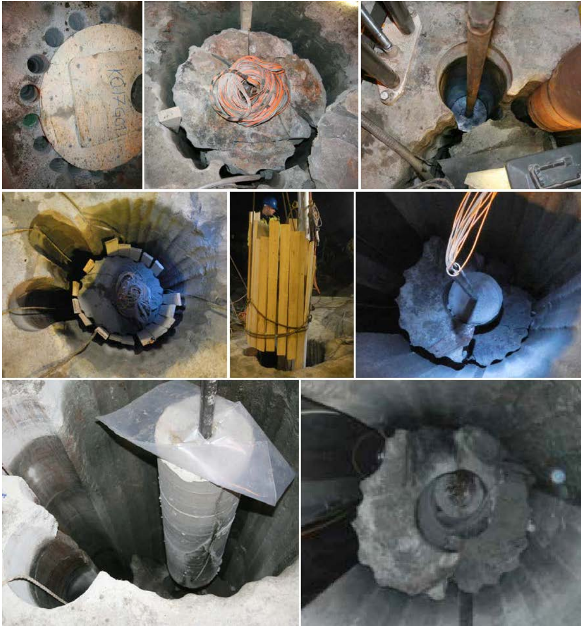
Figure 4-19. Pictures for dismantling of parcel in Hole 17. On-going stich-drilling (upper left), stich-drilling completed (upper center), core-drilling of \varnothing 250 mm holes (upper right), wire-sawing completed (middle left), lifting of rock piece (middle centre), remaining bentonite parcel and rock blocks (middle right), pulling of parcel (bottom left), remaining rock blocks (bottom right).
