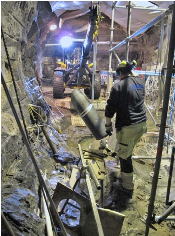
Figure 3-32. TASSO-tunnel (Phase 3) and the ongoing drilling of one of the central 300 mm boreholes.
