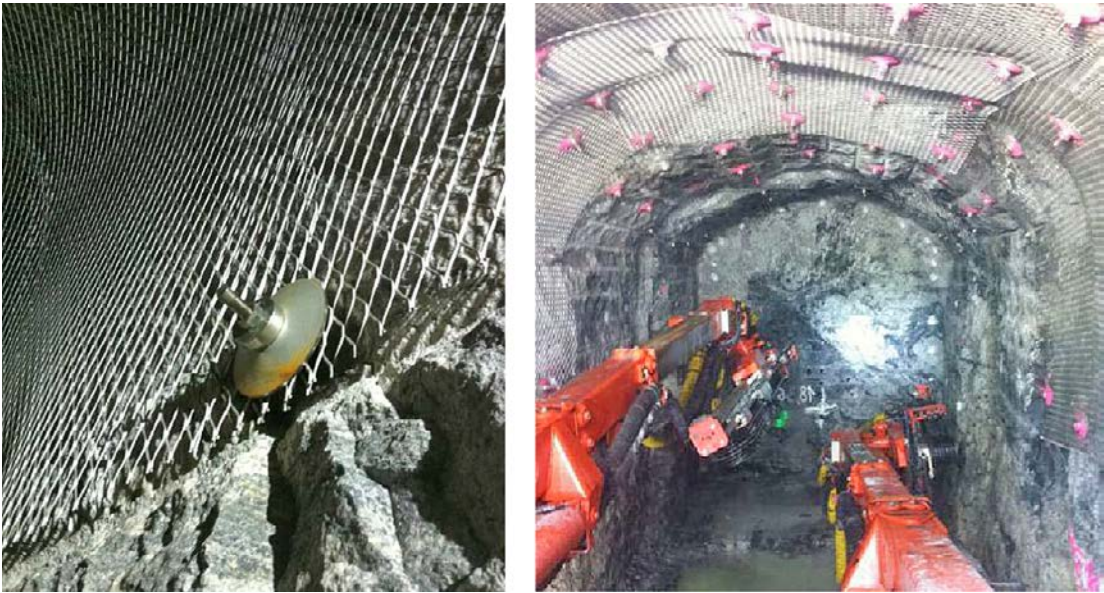
Figure 7-7. Detail of the stainless steel mesh (left) and drilling under reinforced roof (right). After excavation of the next round new mesh is to be installed.
