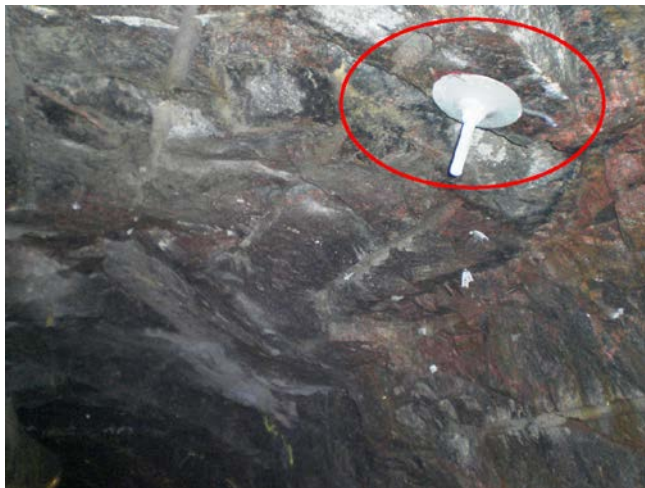
Figure 3-6. Example of a spot bolted potentially loos wedge in the tunnel roof (marked in the figure).
