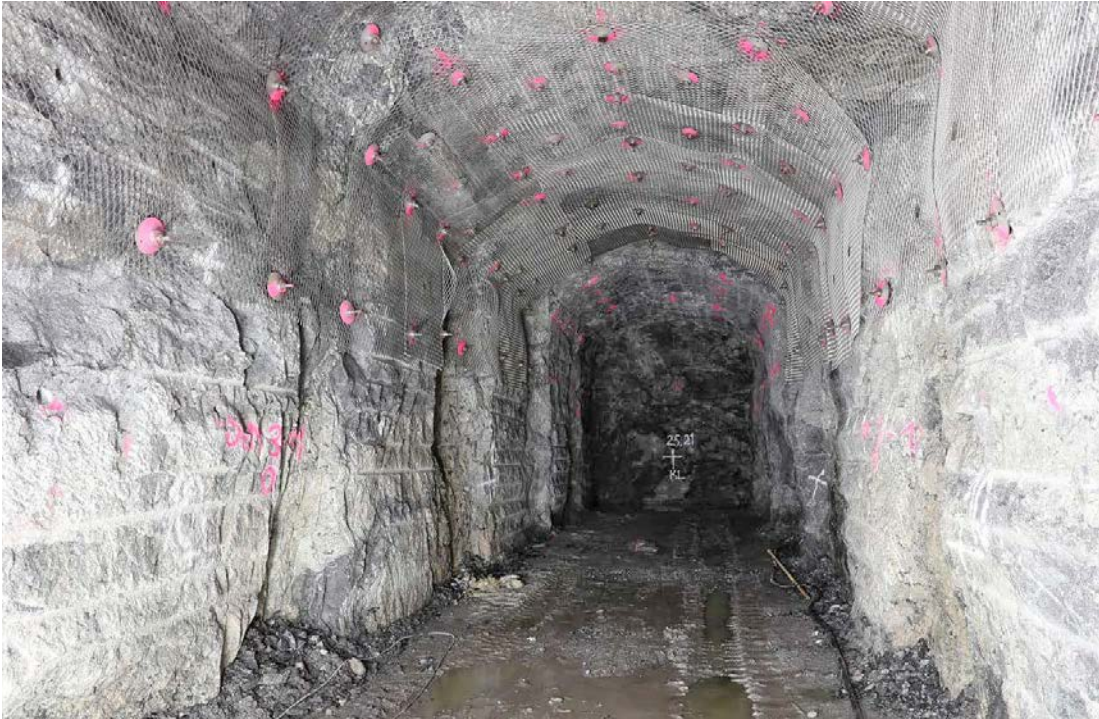
Figure 7-6. Stainless steel mesh and systematic bolting in Demonstration tunnel 3. The bolts are 3 m long.
