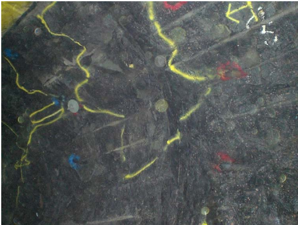
Figure 3-9. Overbreak in the area between two blast rounds. The area boundary is marked with yellow spray paint.
