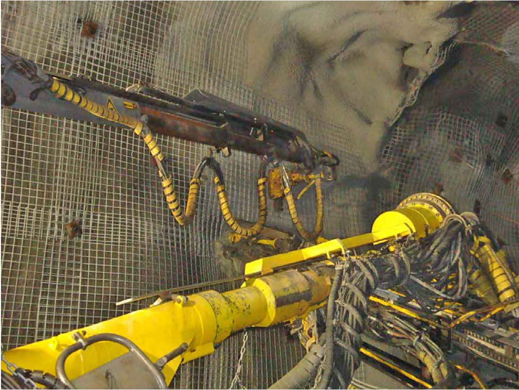
Figure 7-3. Installation of welded wire mesh with an Atlas Copco Boltec rig. The upper boom is holding the mesh with an electromagnet and the lower is installing a swellex rockbolt.
