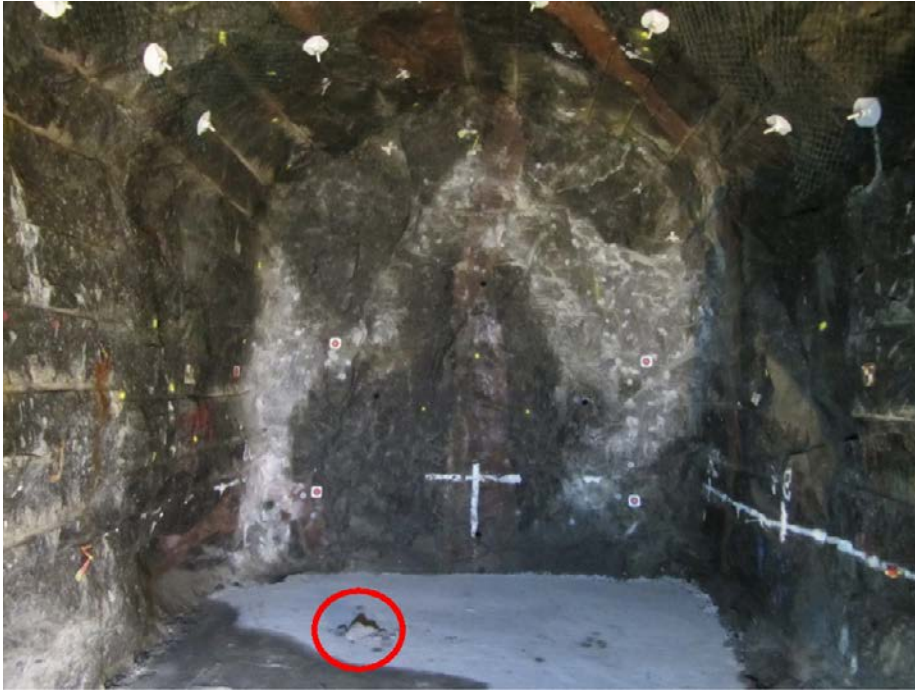
Figure 3-10. Example of fall of ground in the last blast round of the TASS. The block is marked with a red circle in the figure. It originated close to a section supported with chain linked wire mesh.
