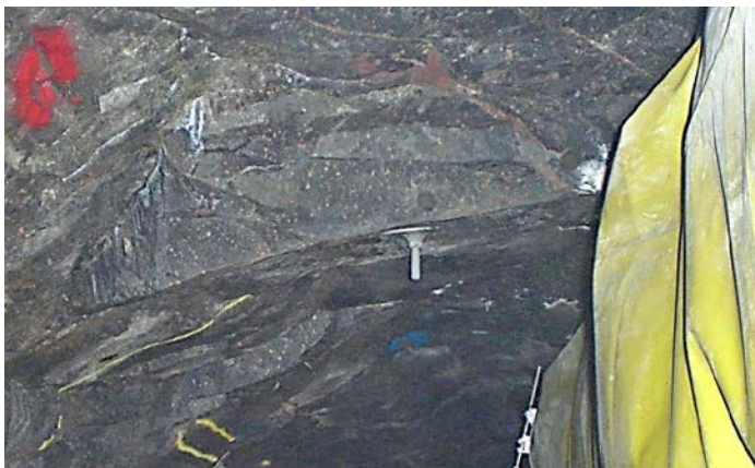
Figure 4-13. Deviation in geometry in the end section of a blast round. Note the block supported with a rock bolt.
