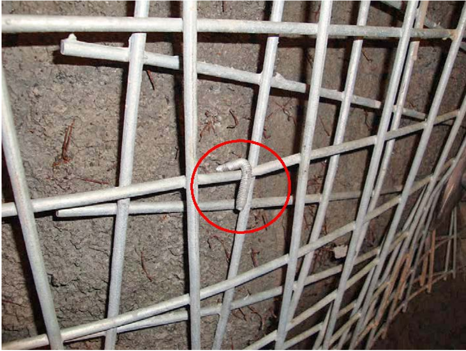
Figure 7-4. Welded wire mesh, temporary holed in place with a hand drilled fastener, marked with a red circle in the figure.
