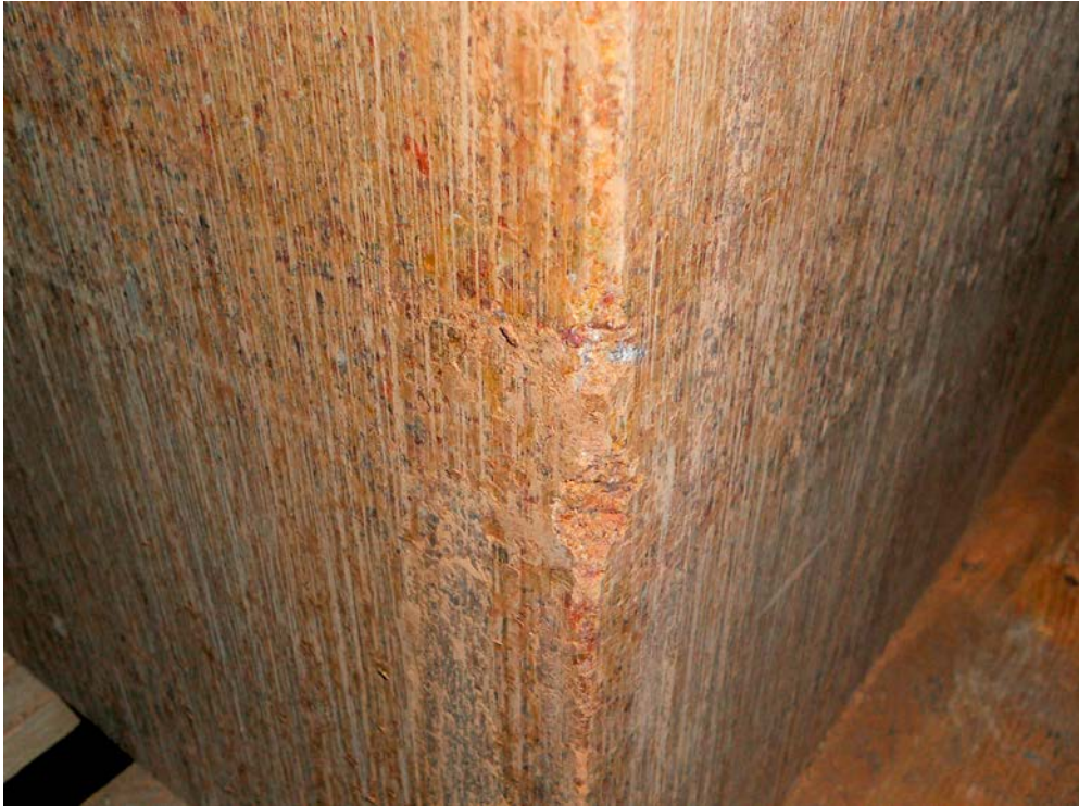
Figure 2-6. Brittle edges on a backfill block.
