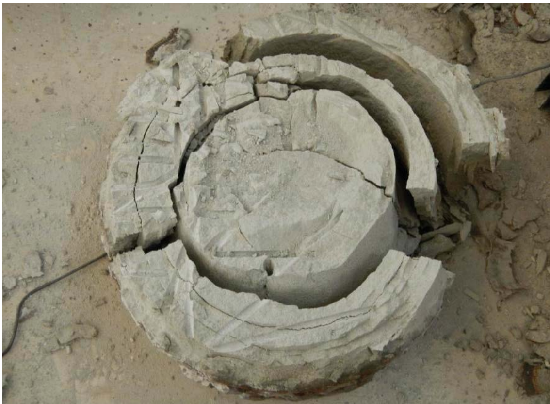
Figure 2-20. BB II, cross section C. A layered structure was revealed when a large block part fell to the floor.
