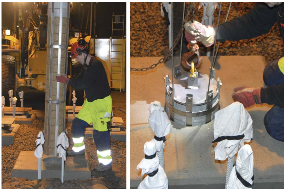
Figure 9-3. Installation of a package with 30 bentonite blocks. Each block also contains four smaller material samples.
