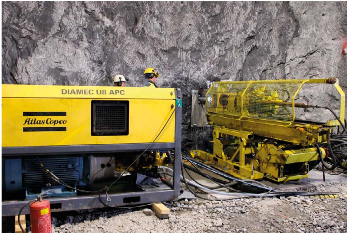
Figure 4-7. The Atlas Copco B20 APC drill rig at the ONK-PH 28 drill site. The powerful drill rig stands on a solid concrete platform surrounded by hard-packed gravel. To the left the electrically powered hydraulic unit is shown.
