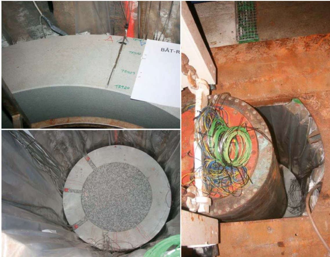
Figure 4-41. Fotos from the installation. Uppder left: installation of sensors in buffer blocks, lower left: Top buffer ring. Right: installation of canister:
