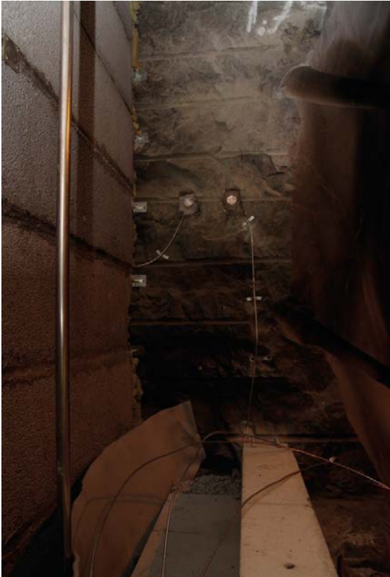
Figure 4-34. Detail photo showing (from left) delimiter of leca-beams, gravel filter with drainage (air) pipe, delimiter of geotextile, bentonite seal of MX-80 (blocks and pellets) and delimiter of concrete beams. All sensor cables are led in steel tubes.
