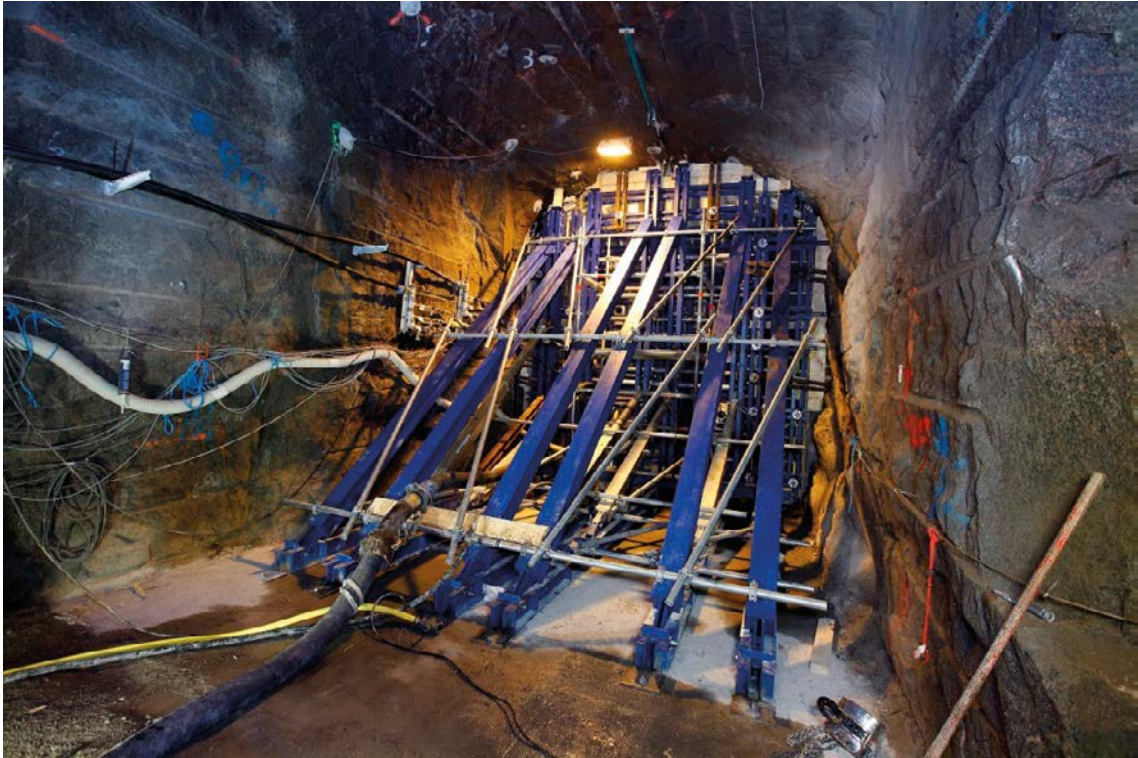
Figure 4-36. Concrete is pumped in behind the formwork for casting of the concrete dome structure.
