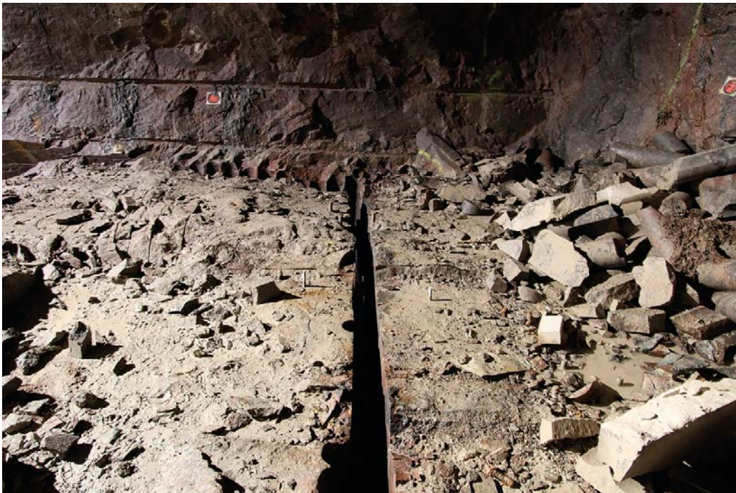
Figure 4-45. Completed slot next to the tunnel face. Parts of the slots were excavated by seam drilling, see upper part of the photo (Photo by Rickard Enér).
