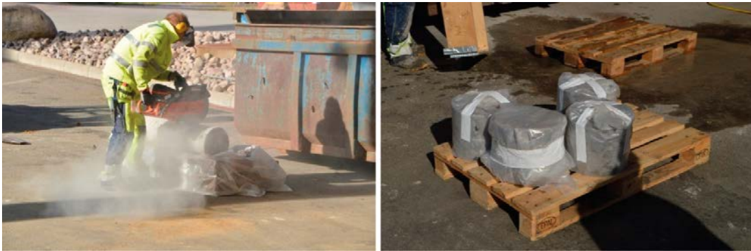
Figure 4-20. The concrete cylinder was cut into four different pieces, each containing only one type of metal specimens, packed and shipped to CBI for analysis.
