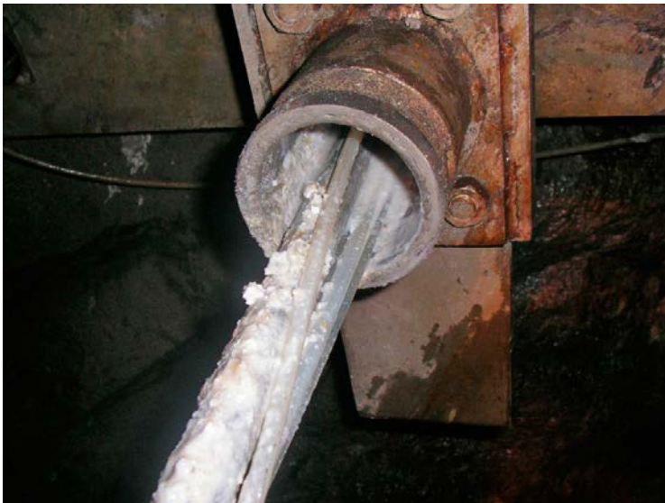
Figure 3-3. The upper part of the existing equipment (near the tunnel wall) when it was removed from the borehole. The white coating is oxide.
