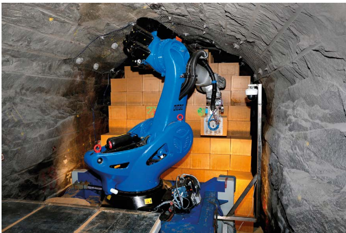
Figure 8-4. Installation robot operating in the TASS-tunnel.
