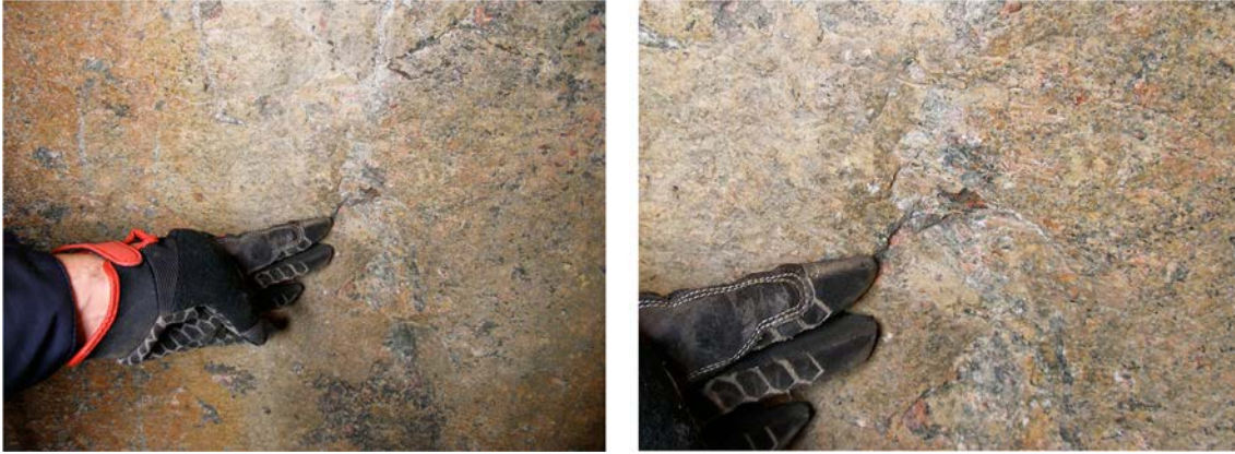
Figure H-2. Illustration of potential damage to the wall in Hole 6. This area is located approximately at the position marked with the shaded area "9" in Figure H-1 (right). Right: Close-up of left figure.
