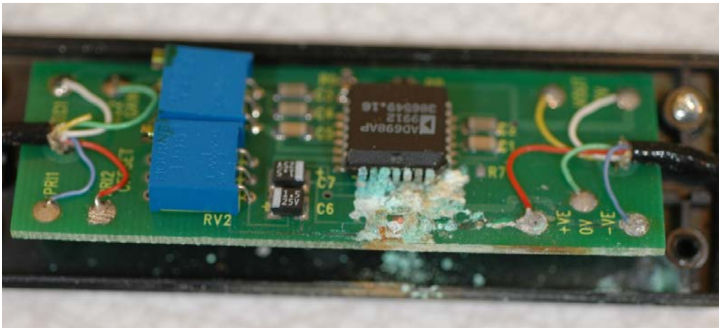
Figure D-4. Electronics of displacement sensor 1.
