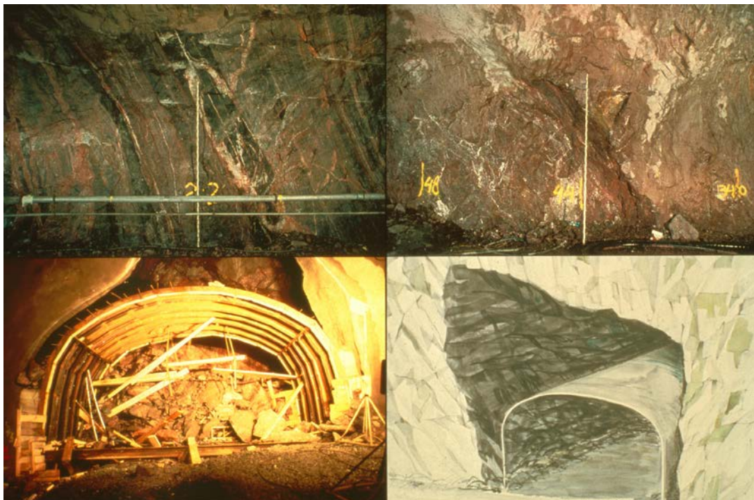
Figure 4-15. Illustration of the difference in rock mass conditions within the Singö Deformation Zone between Forsmark 1 and 2 tunnel (upper pictures) and the Forsmark 3 tunnel (lower pictures). (Carlsson and Christiansson 2007, Figure 9-1).
