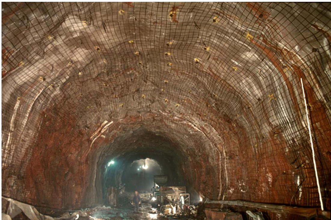
Figure 5-4. Rock support in Ground Type GT4. The wire mesh was later covered by shotcrete, Forsmark 1 and 2 discharge tunnel. (Carlsson and Christiansson 2007, Figure 7-10).
