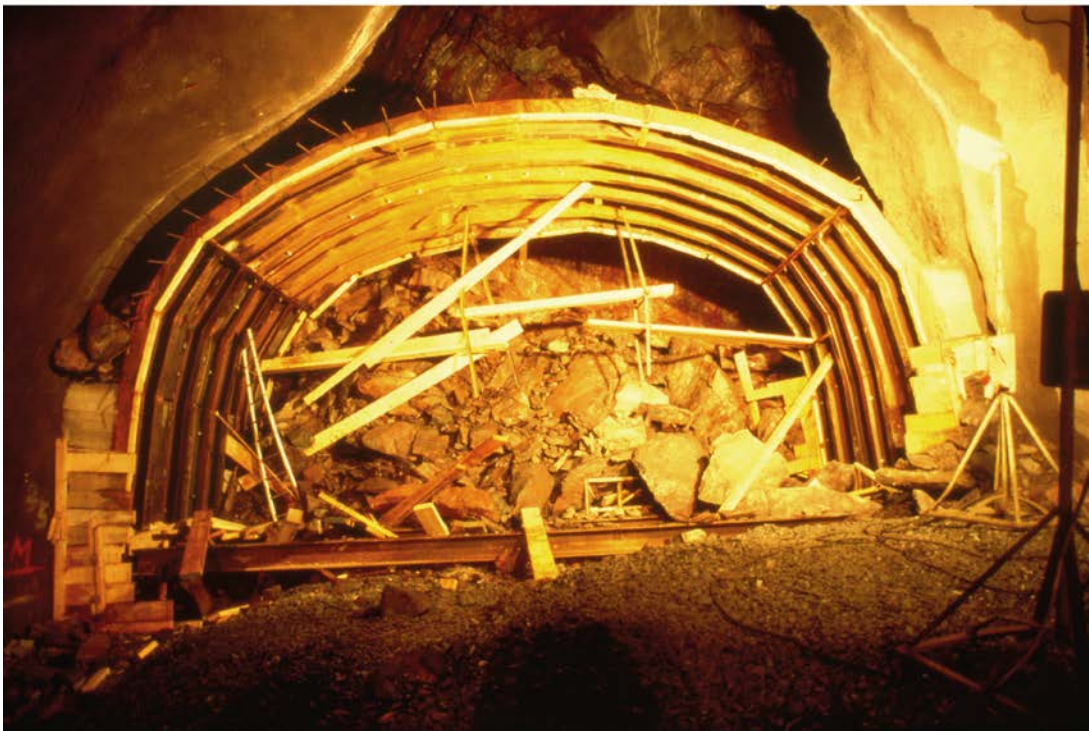
Figure A-3. The steel arch placed in position within the over-break area in section 2/545 in the Singö Deformation Zone, Forsmark 3 tunnel. b. Further rock fall occurred after the erection of the steel arch; section 2/545 in the Singö Deformation Zone, Forsmark 3 tunnel. (Carlsson and Christiansson 2007, Figure 4-11).
