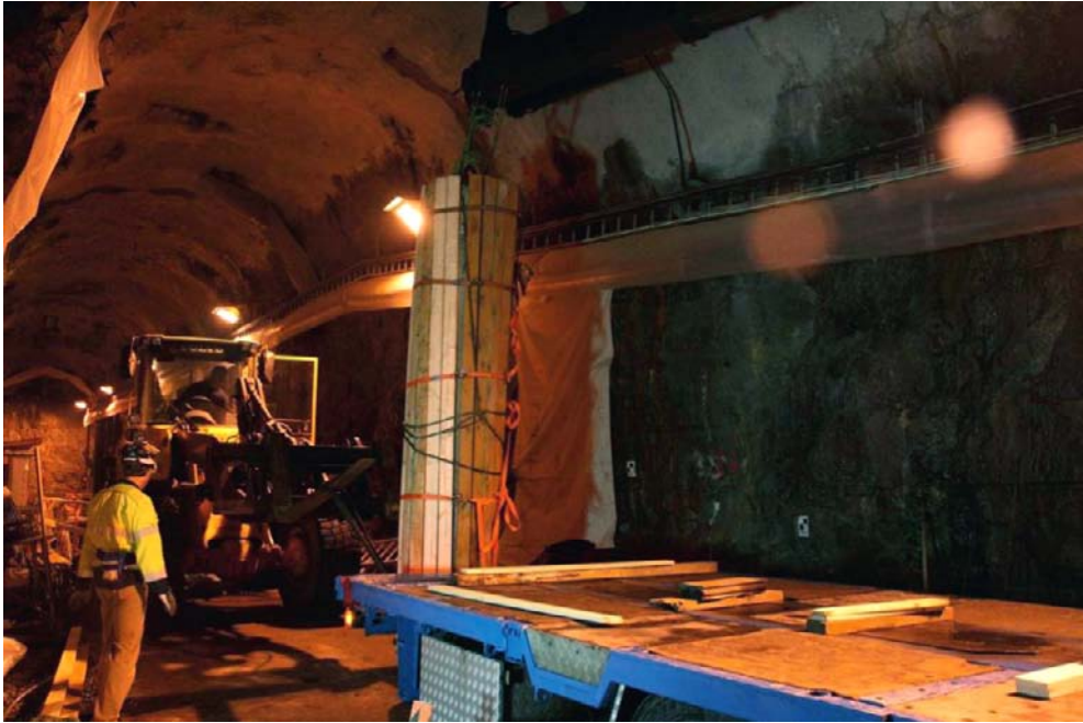
Figure 5-7. The test package was lifted up in one piece. In order to avoid pieces from falling off during the handling, the test package was surrounded by boards and straps.
