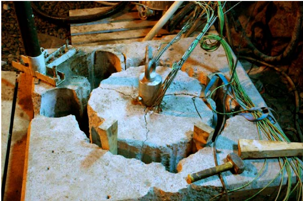
Figure 5-6. Photo showing the released test package. After the seam-drilling, two core drilled holes with a diameter of 300 mm were drilled in order to make it possible to install the wire-sawing equipment and saw off the rock column in the bottom.
