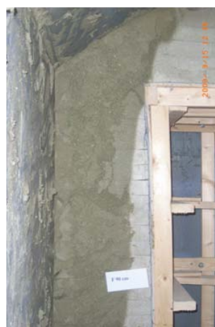
Upstream of fracture, extensive block wetting
