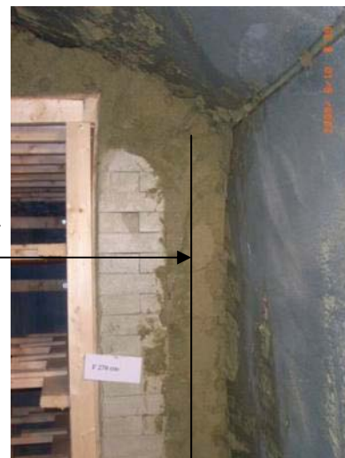
60 cm downstream from fracture block wetting is not as extensive
