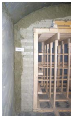
Block wetting at fracture location
