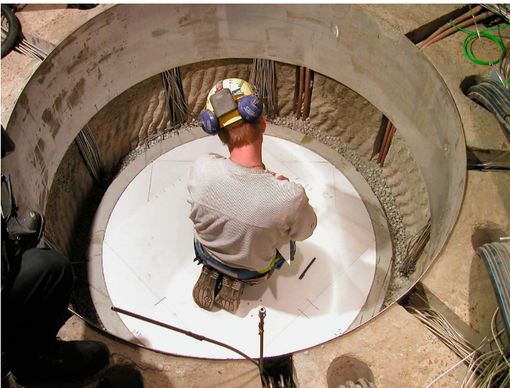
Figure 8-10. The outer gap between block C4 and the wall of the deposition hole filled with pellets of MX-80.
