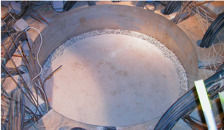
Figure 8-9. The filter consisting of two layers placed on top of block C3.
