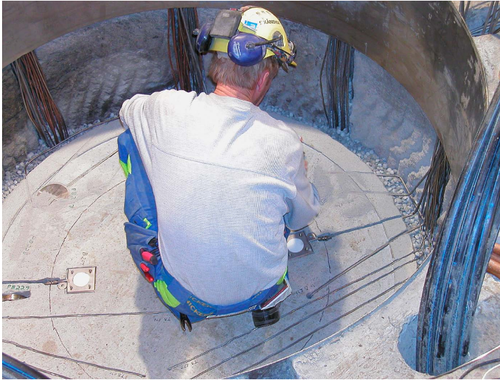
Figure 8-8. The two plates used for applying the filter with water placed on the surface of block C3.
