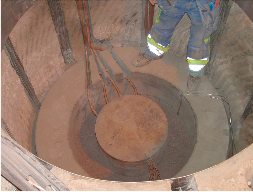
Figure 6-5. The upper heater placed in the deposition hole before the inner gap (the shield) was filled with sand.
