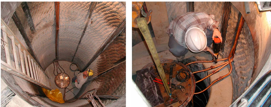
Figure A4-11. Protection tubes installed along rock slot in lower heater (left) and detail of installation in upper heater (right).
