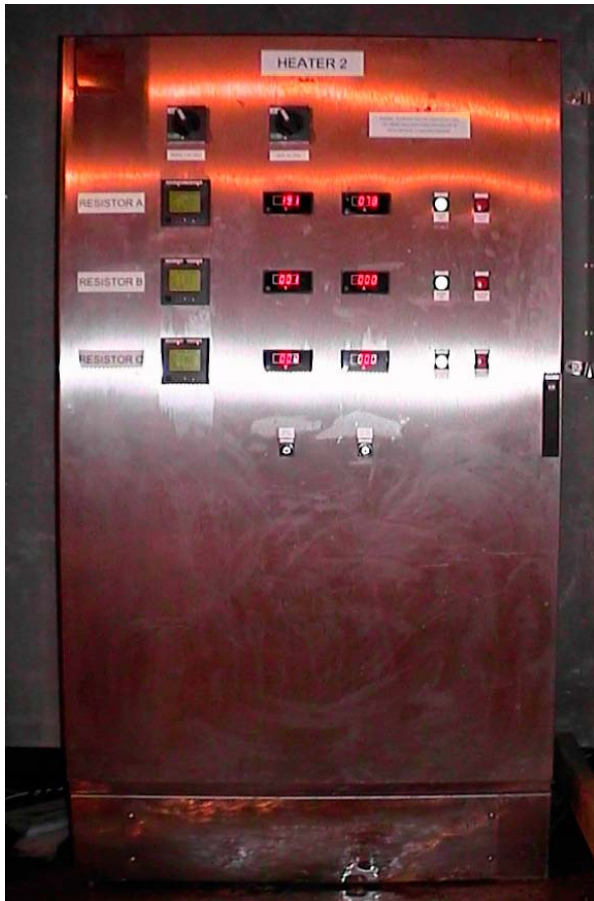
Figure A4-13. Power regulation cabinet for heater 2 with PID modules.
