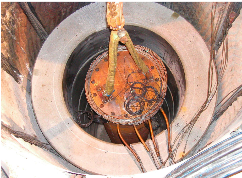
Figure 8-4. The upper heater placed in the deposition hole.
