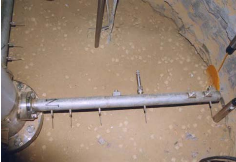
Figure 2-8. Pellet – clay material installed in Reseal Project's field demonstration (Gens et al. 2009).
