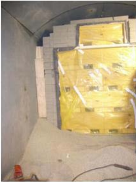
Figure 2-6. Placing dry Cebogel QSE pellet materials into space between backfill blocks and chamber wall in 1/2-Scale Experiment at Äspö. (Note slumping of pellets and need to install temporary wooden wall to keep dry pellets in place).
