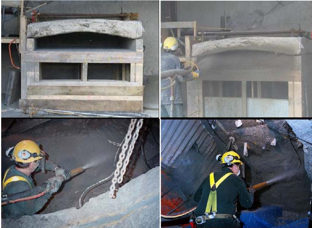
Figure 2-10. Installation of bentonite-based LBF materials to fill rough-surfaced mock-up and real excavation at 420 m level at AECL URL. Upper: backfilling of a simulated deposition tunnel roof section (Martino and Dixon 2007); Lower: installation of bentonite-aggregate filler materials to provide a continuous contact between rock and clay blocks in AECL's Tunnel Sealing Experiment (Chandler et al. 2002, Martino et al. 2008).
