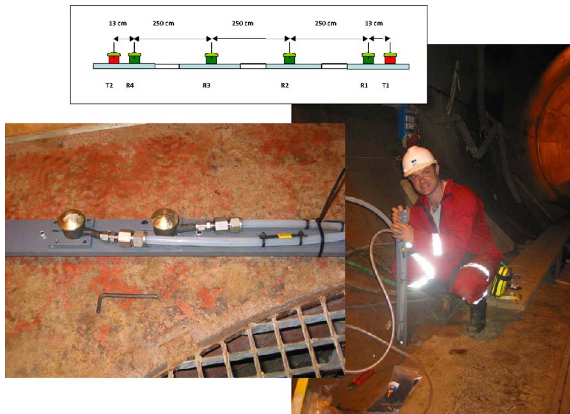
Figure AII-1. Top: Schematic diagram of the locations of all transducers on a single frame. Left: Photo of a section of the transducer assembly. Right: Transducer assembly during installation.
