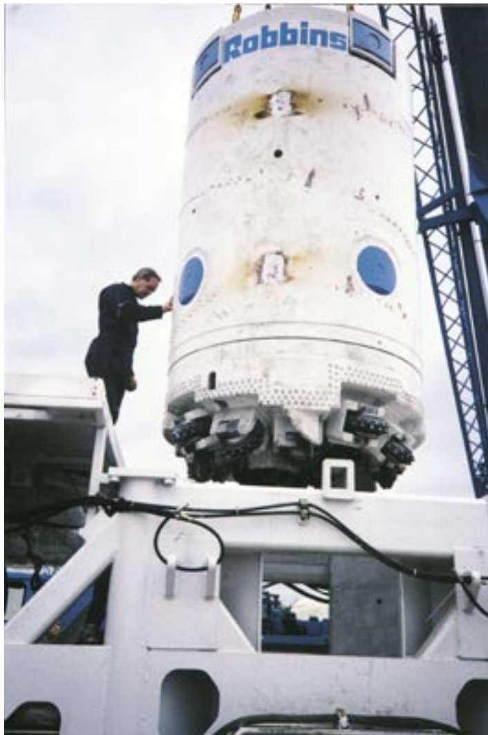
Figure 4-30. Photo on the Shaft Boring Machine used to drill test deposition holes at Äspö HRL.
