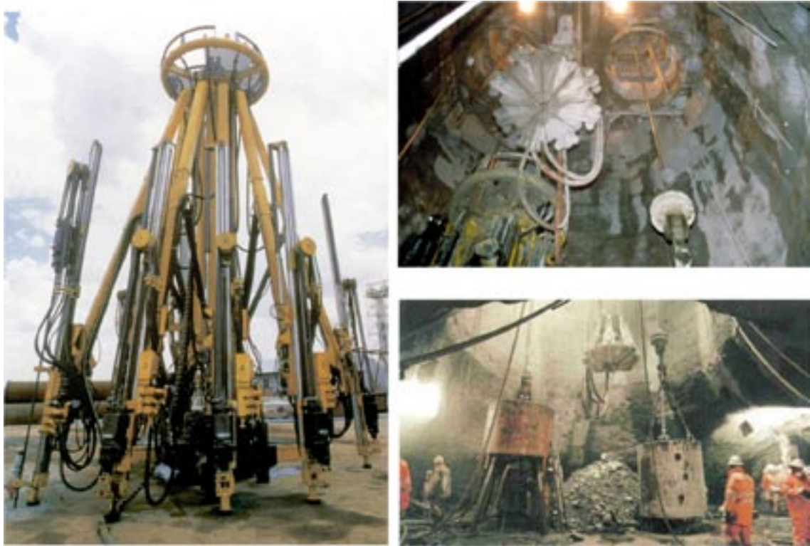
Figure 4-2. Pictures from equipment at shaft sinking in Sedrun, Switzerland. Drilling rig with 8 booms (left). View up from the shaft floor (top, right). Mucking equipment with grippers and bucket (down, right). Courtesy: Electrowatt Infra.
