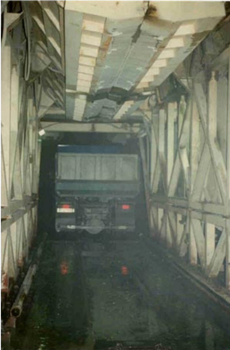
Figure 4-18. Photo from truck that removes muck from the belt-conveyor at the TBM-project in Bergen. Photo: Courtesy Odd G Askilsrud.
