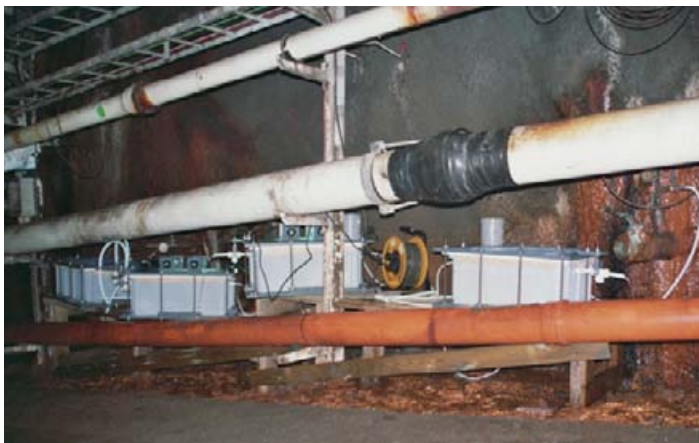
Figure 7-6. Flow reactor set (white boxes) installed at TASA 1327B in 2006.
