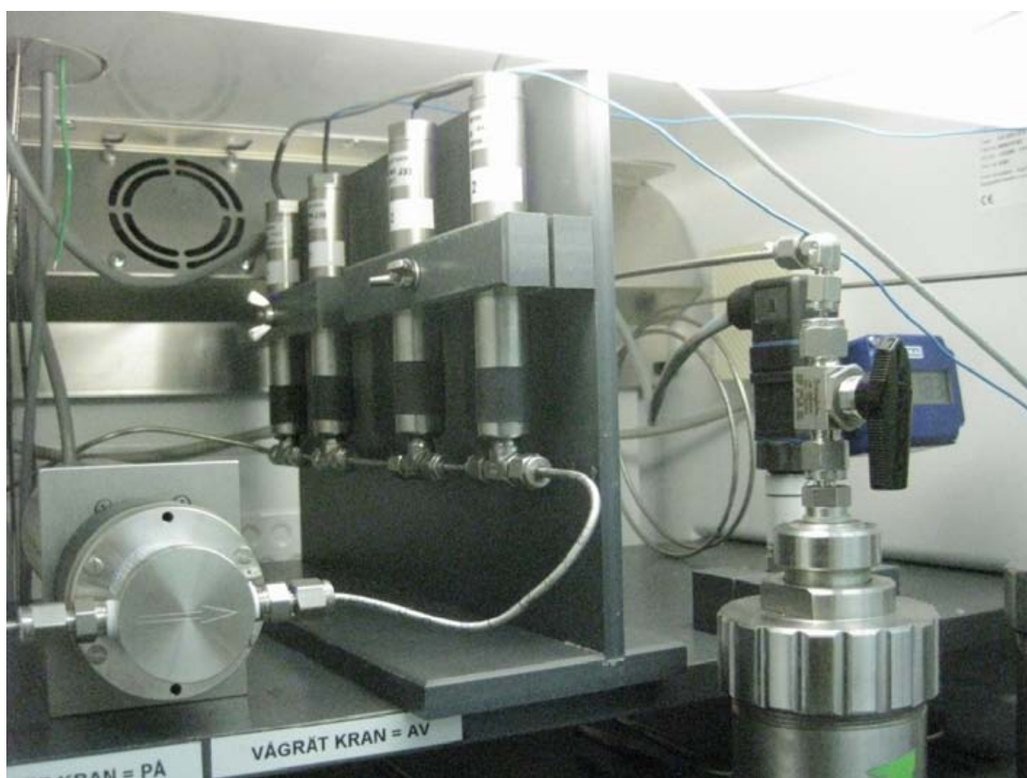
Figure 3-7. Two pairs of pressure resistant redox electrodes installed on-line on the circulating groundwater in one of the stainless steel circulation systems.
