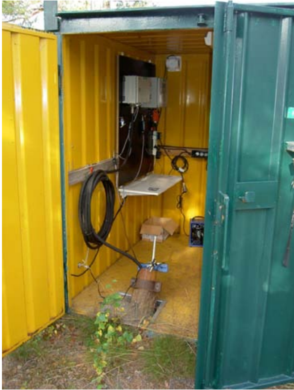
Figure 2-5. Typical housing of monitoring equipment as exemplified with container at borehole KAS04.
