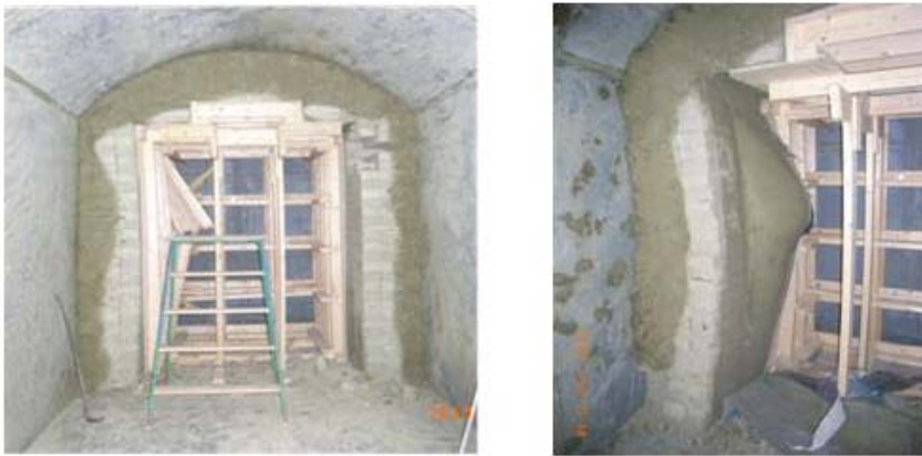
Figure 6-3. Wetting at/near inner fracture feature showing location of restraint failure and subsequent clay swelling.
