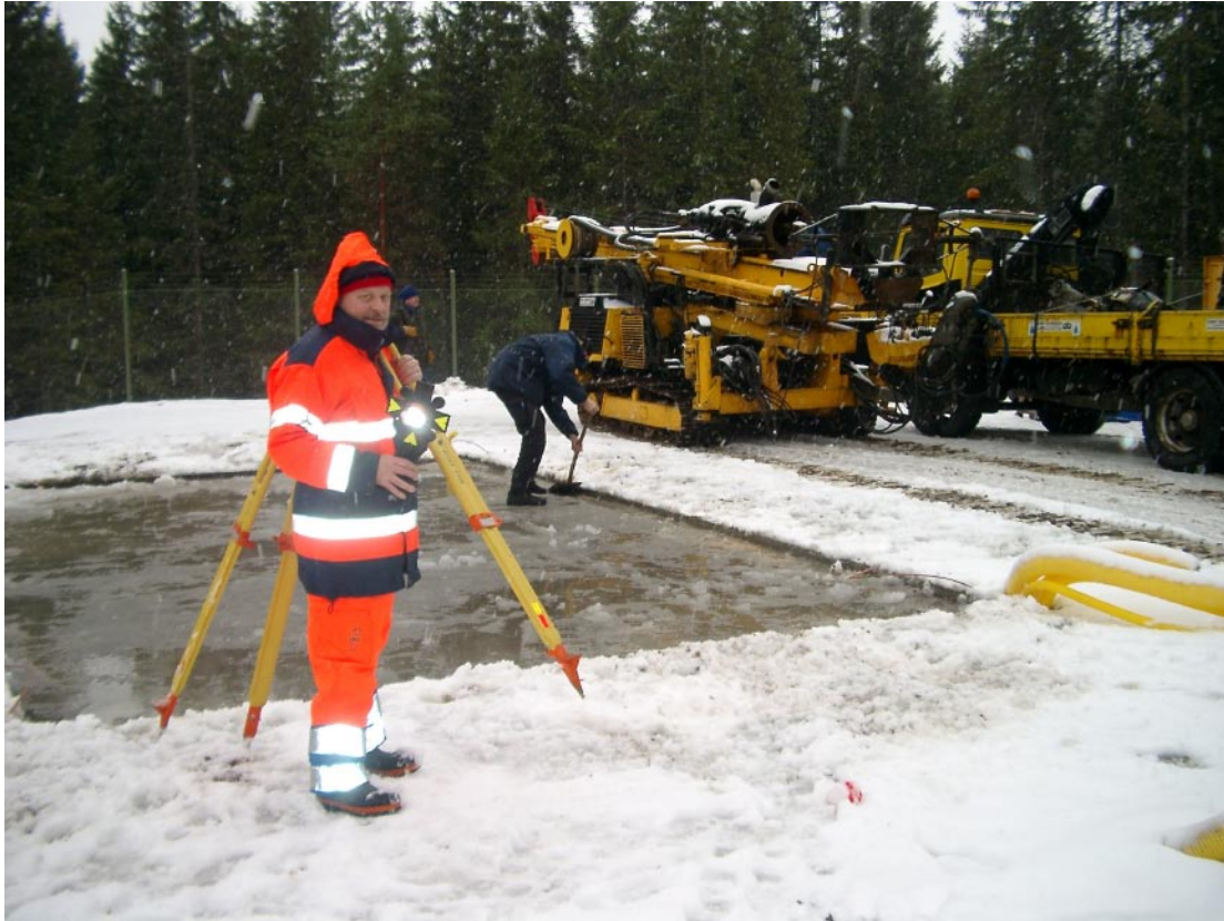
Figure 4-1. Lining up the drilling machine was made with the help of a theodolite.
