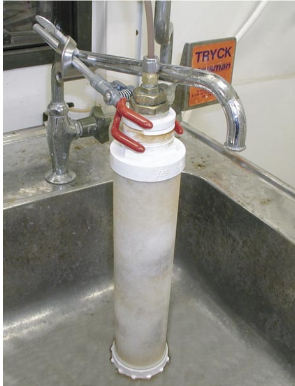
Figure 4-5. The ion exchange column mounted to the outlet of pumped groundwater from the borehole section.
