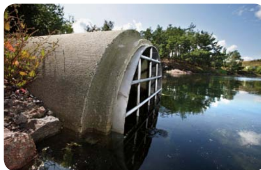
Figure 8-6. Discharge pipe from the sewage treatment plant at Hamnefjärden.
