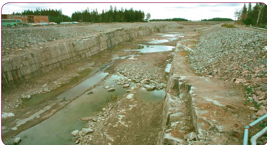
Figure 7-11. Example of what horizontal water-conducting fractures in fracture domain FFM02 look like near the surface. Photo taken during construction of the cooling water channel in Forsmark.
