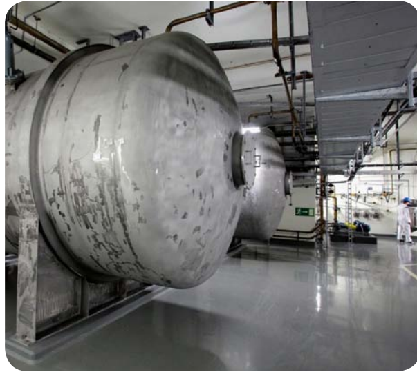
Figure 8-4. Collection tanks for process water at Clab.
