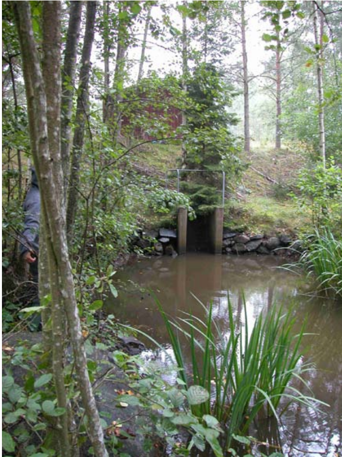
Figure 4-33. Pumping station in the Söråmagasinet reservoir pumping freshwater into the reservoir from Laxemarån.
