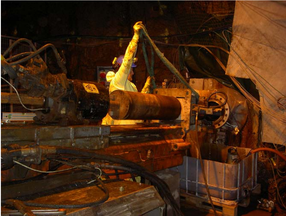
Figure 3-6. Drilling machine is prepared for 300 mm diameter over-core drilling at experimental borehole KA3065A03. Drill bit with core barrel in centre of photo. Open vessel for collecting drilling fluid beneath borehole collar.
