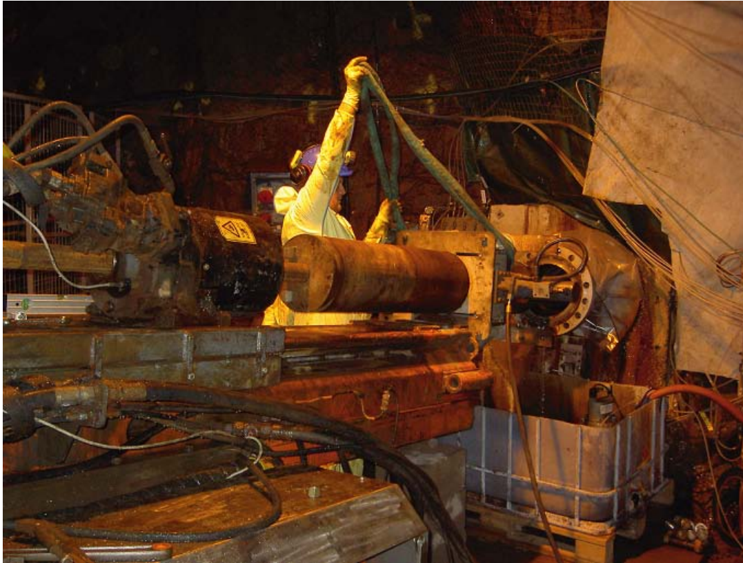
Figure A2-2. The drilling machine is prepared for 300 mm diameter over core drilling at experimental borehole KA3065A03. Drill bit with core barrel in centre of photo. Open vessel for collecting fluid beneath borehole collar.
