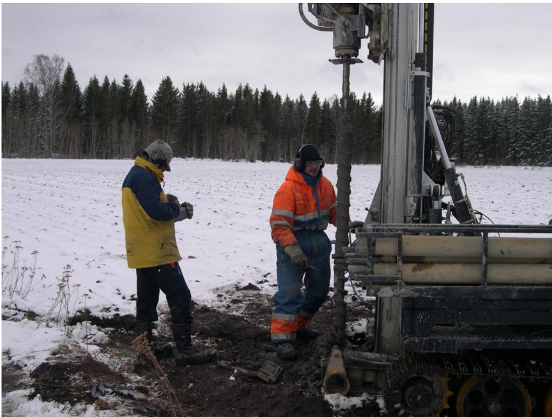
Figure 3-1. The drilling rig Geo Machine GM 100 GTT was used for drilling and sampling. Nils Lindqvist and Mesgena Gebrezghi from Sweco VBB Viak was operating the drill rig.
