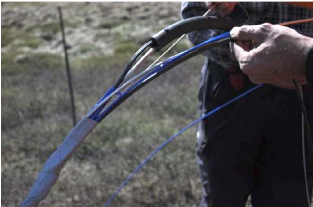
Figure 4-22. Photo of the deployment string, i.e. tubing and cables attached to the top of the borehole observatory. DTS cable (blue), sampling tubing (stainless steel), heater cable (black), P/T/EC sensor cable (black with blue tape). The black insulating jacket is also shown. Photo by Lillemor Claesson Liljedahl.
