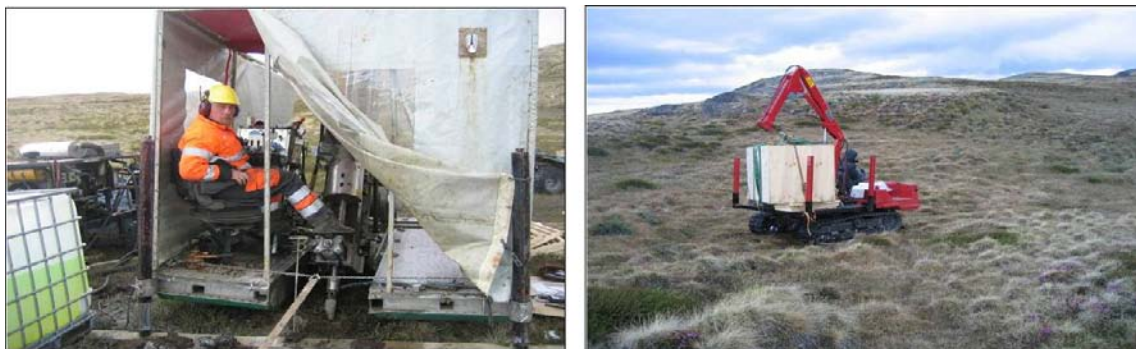
Figure 4-2. Onram 1000 rig and a mini-dumper for moving material. Photo by Timo Ruskeenieni.
