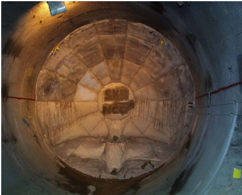
Figure 13-7. Cast plug for the inner section in the Prototype Disposal Tunnel at the Äspö HRL.
