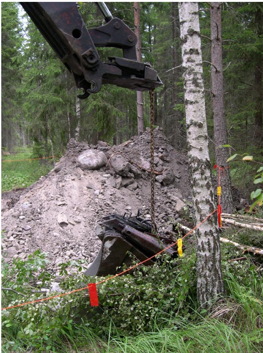
Figure 5-4. The attachment to the excavator bucket broke under the attempts to cut into the extremely hard clayey till (PFM002581).
