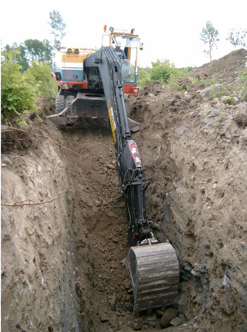
Figure 3-1. Excavator capable to reach depths of c 5 m was used for trenching.
