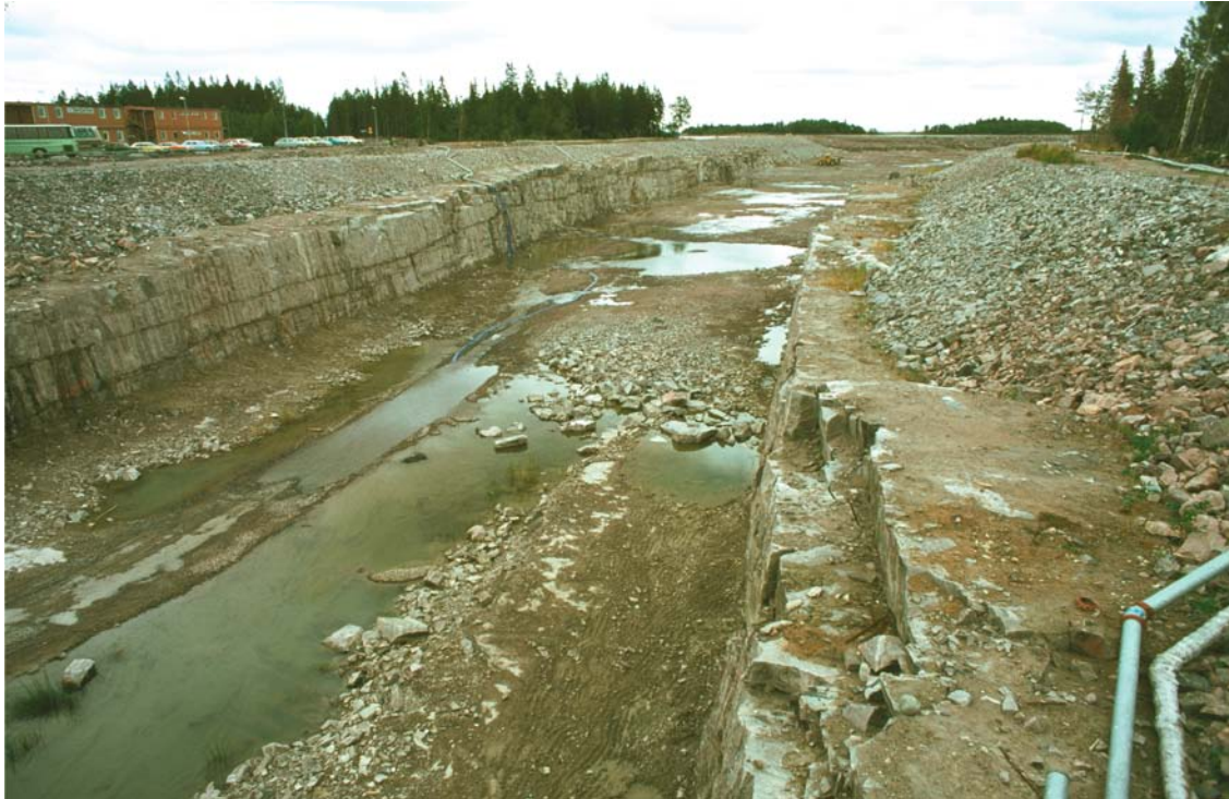
Figure 3-10. Picture from the construction of the 13 m deep and more than one kilometre long canal between the Baltic Sea and the nuclear power reactors in Forsmark. Horizontal fractures/sheet joints are encountered along the entire excavation. The sheet joints follow the undulations of the bedrock surface implying that many of them do not outcrop, but stay below the bedrock surface as this dips under the Baltic Sea. There are several “horizons” of extensive sheet joints on top of each other as determined by the hydraulic interference tests. (Source: Figure 5-14 in /Follin 2008/.)
