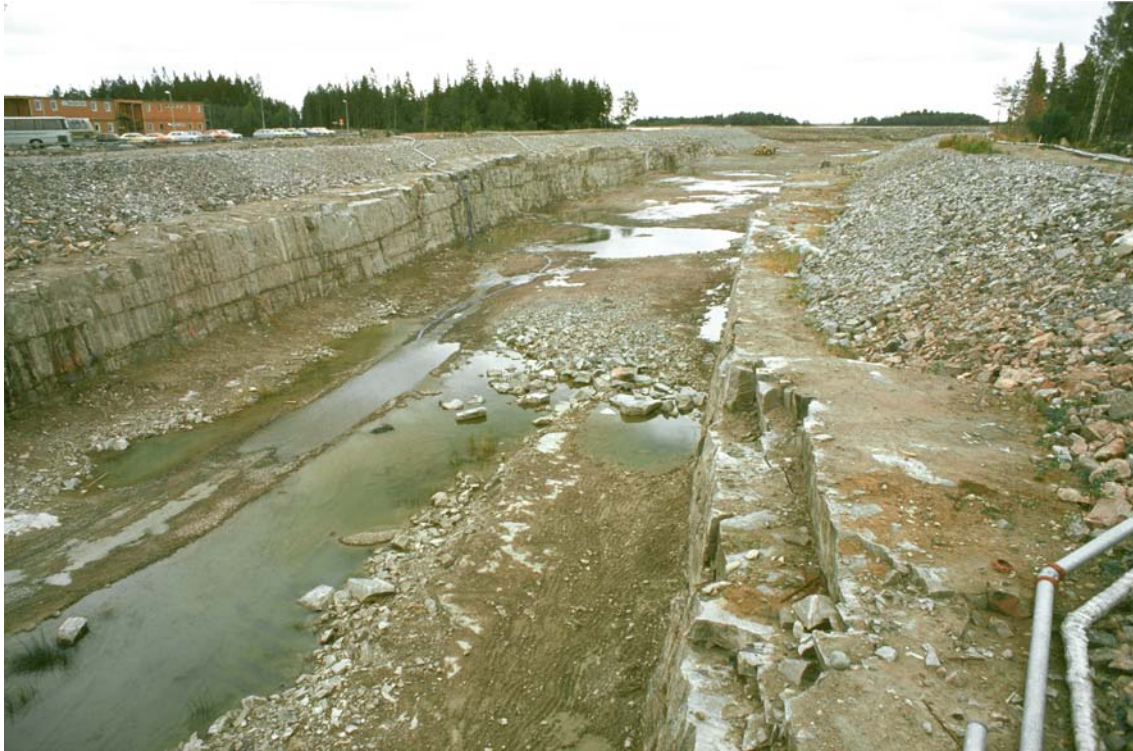
Figure 2-10. Picture from the construction of the 13 m deep and more than one kilometre long canal between the Baltic Sea and the nuclear power reactors in Forsmark. Horizontal fractures/sheet joints are encountered along the entire excavation. The sheet joints follow the undulations of the bedrock surface implying that many of them do not outcrop, but stay below the bedrock surface as this dips under the Baltic Sea. There are several “horizons” of extensive sheet joints on top of each other as determined by the hydraulic interference tests. (Source: Figure 5-14 in /Follin 2008/.)
