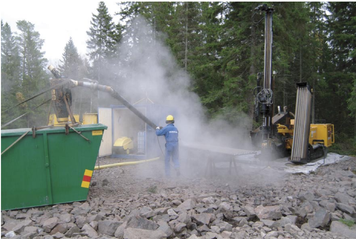
Figure 3-1. The Nemek 407 percussion drilling machine employed for drilling the percussion borehole HFM16 at drilling site DS6. Water and drill cuttings are discharged to the container. The snap-shot illustrates steam-cleaning of drilling pipes.
