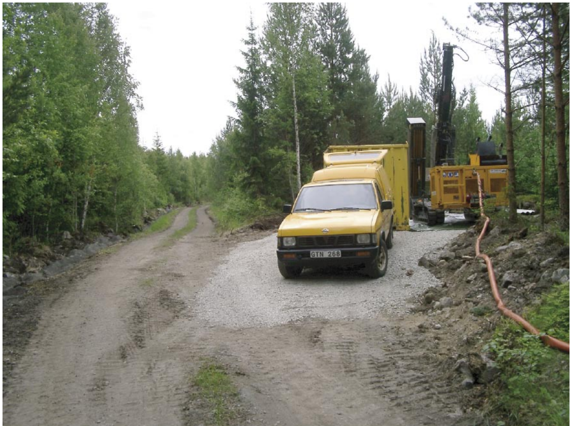
Figure 3-1. The Nemek 407 percussion drilling machine employed for drilling three boreholes at drilling site DS4. Water and drilling debris is discharged to a container.
