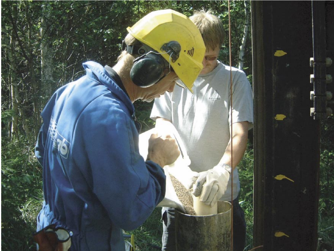
Figure 4-3. Installation of the HDPE well screen, riser pipes, sand filter and bentonite sealings in a groundwater monitoring well inside a temporary steel casing. The snap-shot illustrates when the bentonite is filled between the riser pipe and the temporary steel casing.
