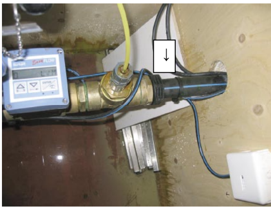
C. Sampling point (2) after UV-unit and tracer addition.
