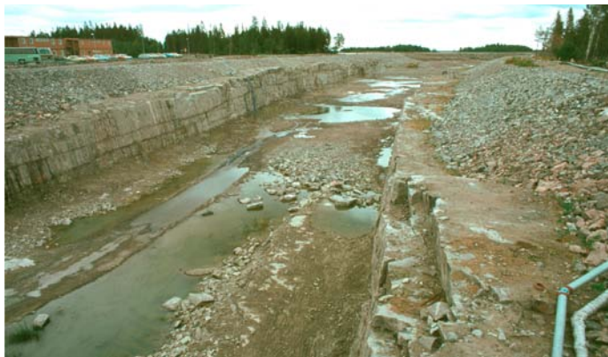
Figure 2-10. Picture from the construction of the 13 m deep and more than one kilometre long canal between the Baltic Sea and the nuclear power reactors in Forsmark. Horizontal fractures/sheet joints are encountered along the entire excavation. The sheet joints follow the undulations of the bedrock surface implying that many of them do not outcrop, but stay below the bedrock surface as this dips under the Baltic Sea. There are several “horizons” of extensive sheet joints on top of each other as determined by the hydraulic interference tests. (Figure 5-14 in /Follin 2008/.)
