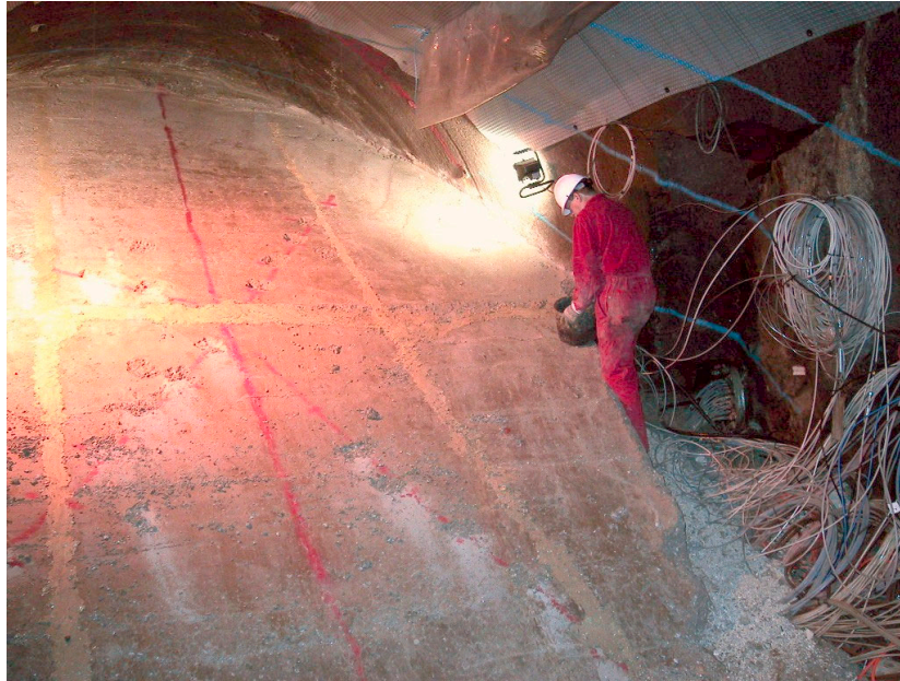
Figure 2-11: Backfill ramp above deposition borehole 6. The electrodes being covered by slightly moistened bentonite powder
