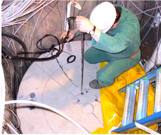
Figure 2-14: Installation of electrode chain in the centre of buffer at top of deposition borehole #5
