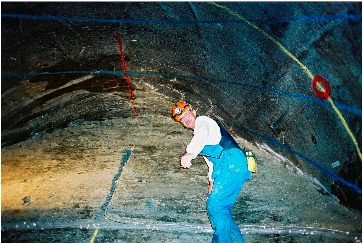
Figure 2-28. The connection of cables and tubes from the boreholes to the lid was made successively during the backfilling operation. Cables and tubes were fixed to the surface of the backfilling before commencing a new layer of backfill material.
