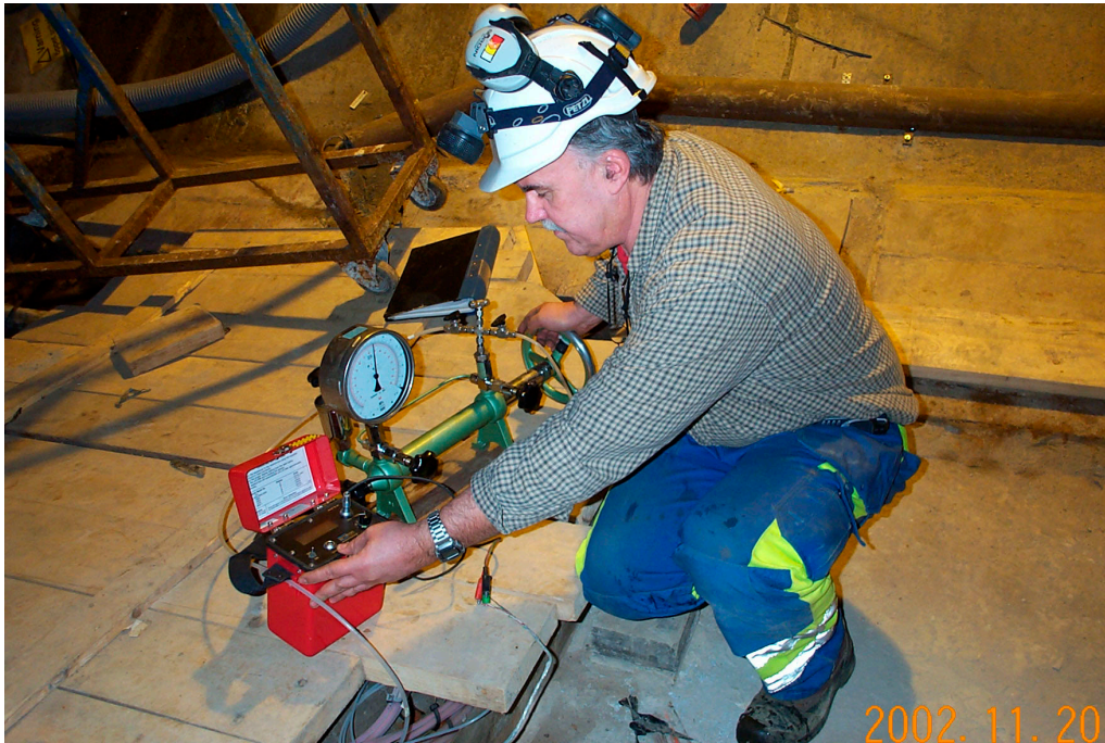
Figure 2-13 During installation of the equipment the positioning and lock cylinders were pressurerised.
