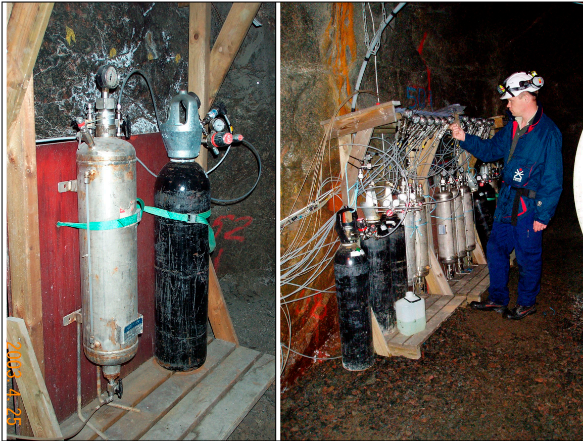
Figure 2-30. The equipment for pressurizing the inflatable packers is in the G-tunnel. A pressure vessel filled with water and connected to several packers. The packers are expanded by pressurizing the water-filled pressure vessel (light above) with nitrogen gas (Nitrogen tube, black above).
