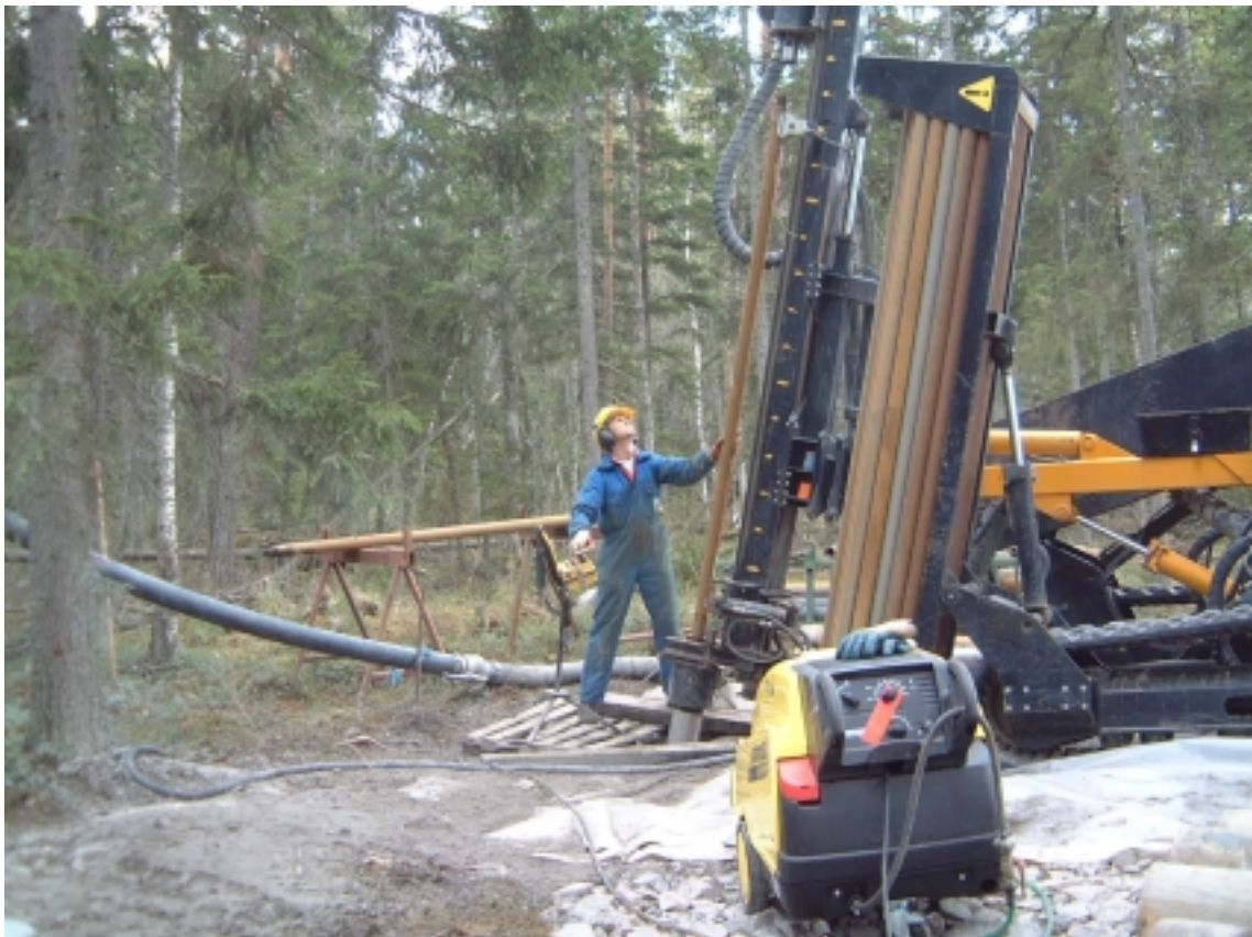
Figure 3-1. The Nemek 407 percussion drill machine engaged for drilling the three percussion boreholes in hard rock at drillsite DS1. Note the fluidproof cover beneath the drill rig used for protection of the ground in case of unintentional oil spillage. Photo Alf Sevastik.
