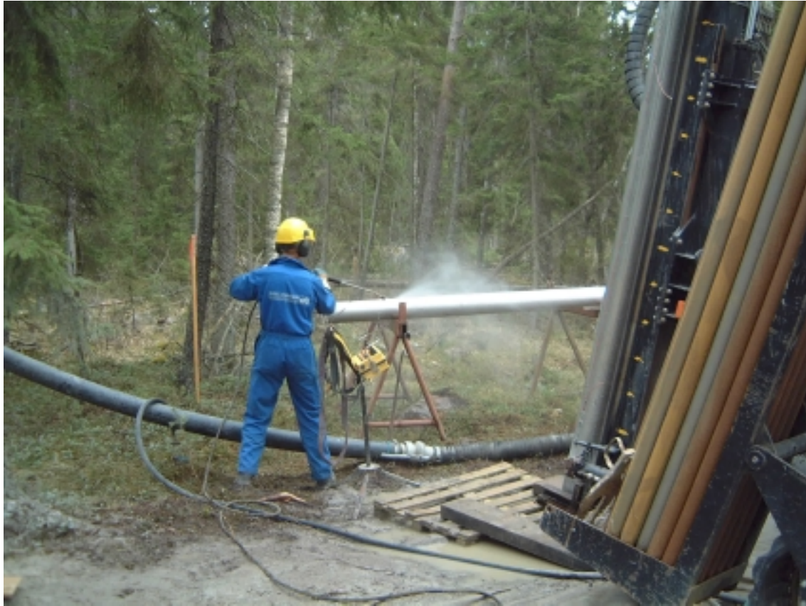
Figure 4-1. A high temperature steam cleaner is used for cleaning the stainless steel casing at level two according to SKB MD 600.004, Version 1.0, before start of Ejector-NO-X drilling. To avoid contamination from surface water and shallow groundwater, the casing is grouted. Photo by Alf Sevastik.
