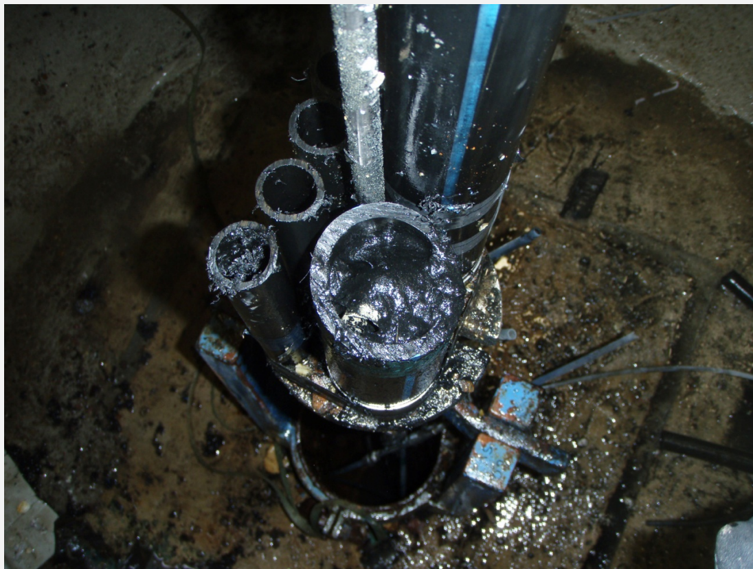
A black precipitate with a smell of hydrogen sulphide in the water standpipes of borehole KAS03. The borehole equipment (iron bars, plastic tubing and rubber packers) was installed more than 20 years ago for groundwater monitoring purposes.
