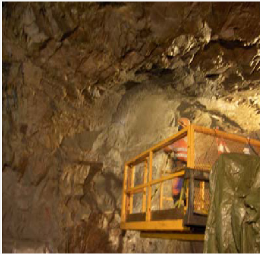
Field test with low-pH shotcrete at Äspö HRL executed within the EC project ESDRED in 2006.
