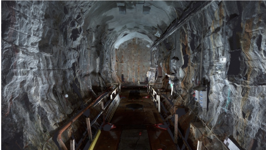
A 3D view of the inner section of the Tasq-tunnel (combination of laser scanning and digital photography).
