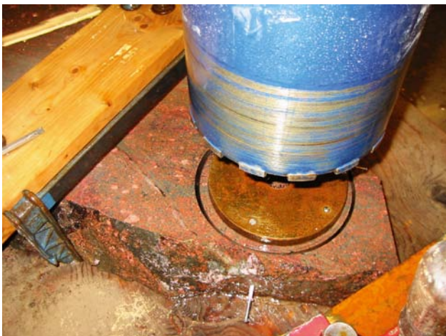
Figure 5-2. Drilling of a larger sample (diameter 200 mm) with a protective steel plate.
