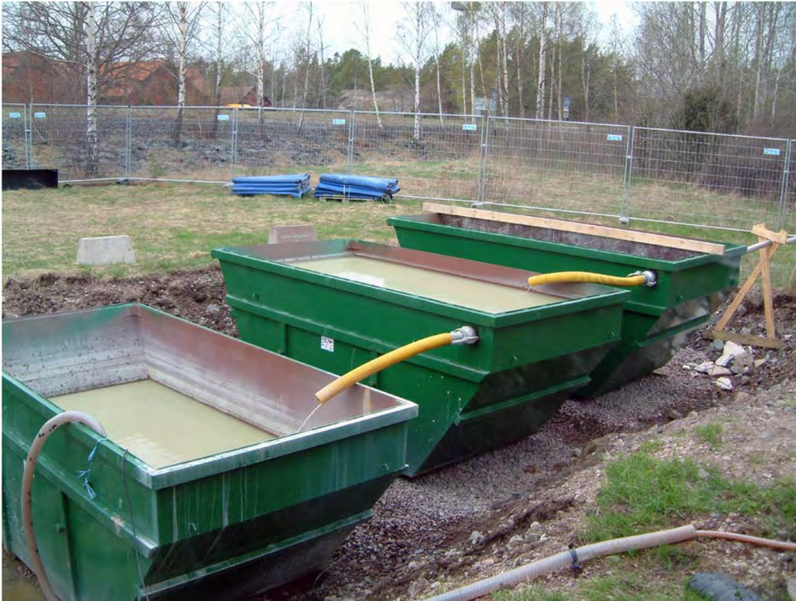
Figure 5-6. The flushing water discharge containers. The sludge and cuttings are allowed to settle in the containers.
