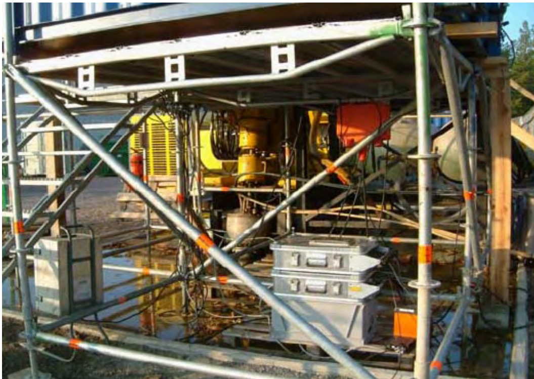
Figure 4-4. The CR23 logging unit for parameters “air-pressure” and “electrical conductivity”.
