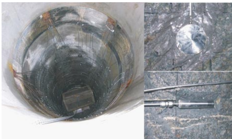
Figure 3-7. The photograph on the left-hand side shows a view looking into the Lasgit deposition hole showing tube work containing the electrical connections from total stress and porewater pressure sensors mounted on rock face. The photographs on the upper and lower right-hand show a total stress and a porewater pressure sensor respectively.
