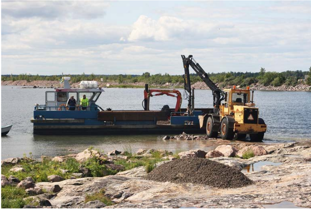
Figure 5-3. Also at the islet “Kobben” a temporary slope was built of gravel carried from the pier with the barge. A bucket loader was stationed on the islet in order to load and un-load the barge.
