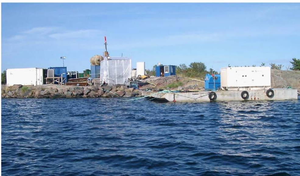
Figure 5-4. The diesel powered electric generator and the fuel tanks were loaded on two sliding barges and anchored beside the KFR106 drill site.
