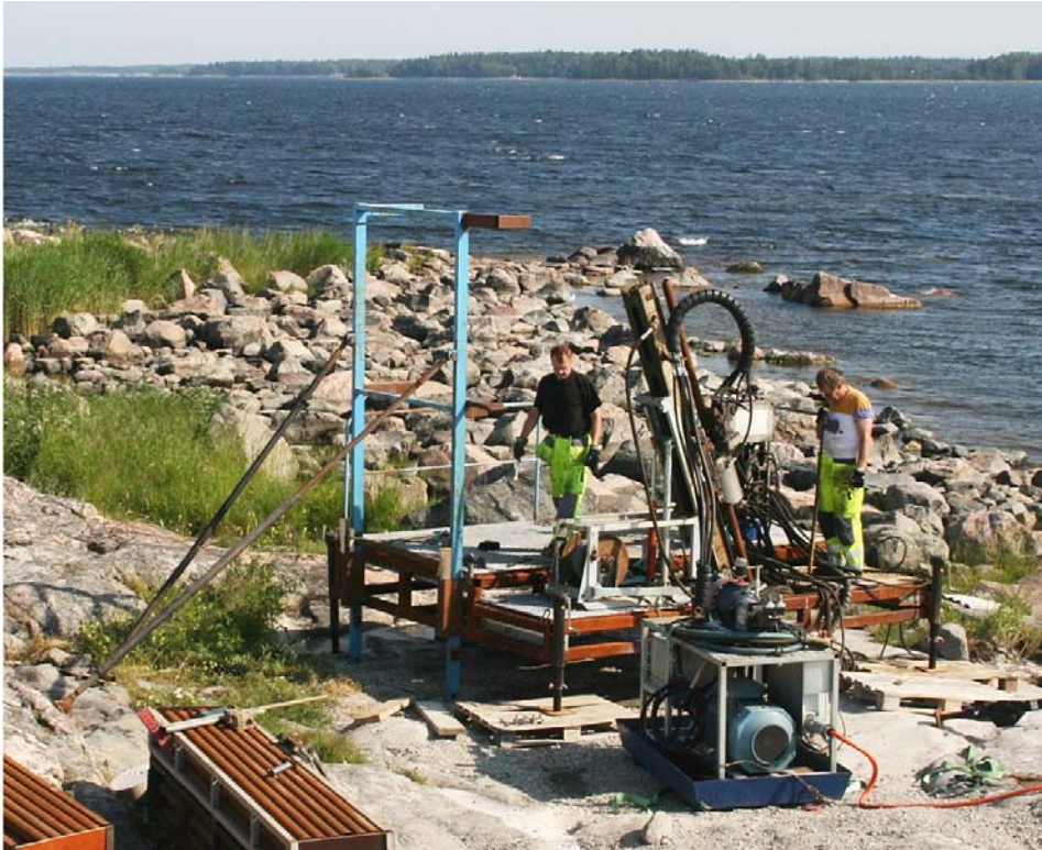
Figure 5-6. Usually, the drilling rig is placed on a concrete plate, but instead, when drilling KFR106, a steel platform was used to fulfil the environmental demands (same platform was used for borehole KFR105 that was drilled from underground).
