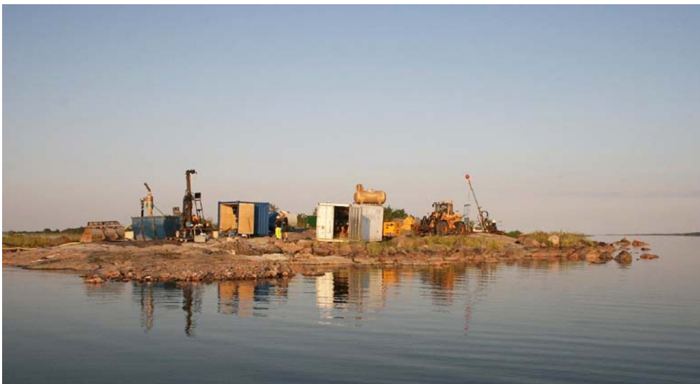
Figure 5-7. Two drilling rigs including all measurement equipment were successfully transported to the islet. To minimize the number of establishments for the flat-bottomed barge, also measurement instruments as BIPS-/radar-, flow logging- and air-flushing equipment were shipped to the islet during the first three weeks.
