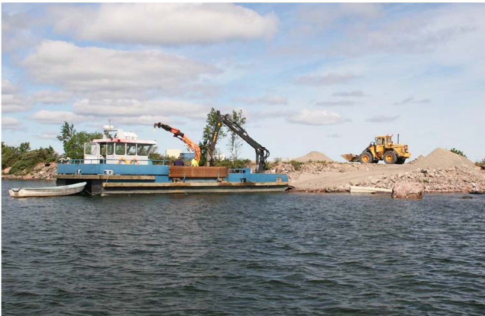
Figure 5-2. At the end of the pier at Asphällskulten a temporary slope was built in order to easily load or un-load the barge.
