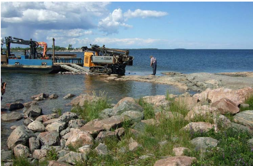
Figure 5-4. The percussion drilling rig arrives to the islet. The air-compressor was left on the pier and supports the rig through a hose floating on the water.
