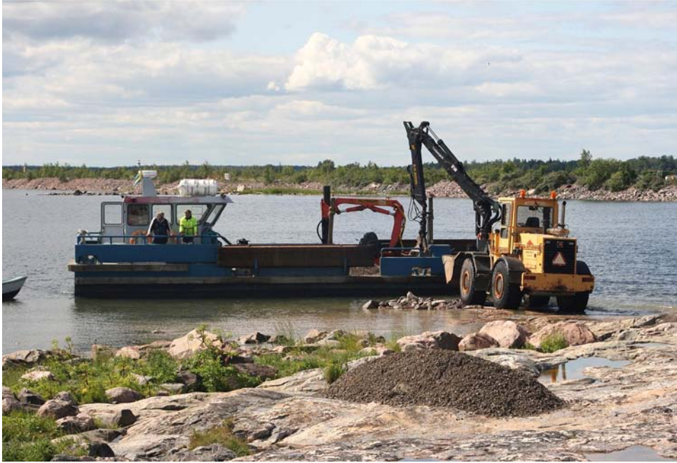
Figure 5-3. Also at the islet “Kobben” a temporary slope was built of gravel carried from the pier with the barge. A bucket loader is stationed on the islet in order to load and un-load the barge.
