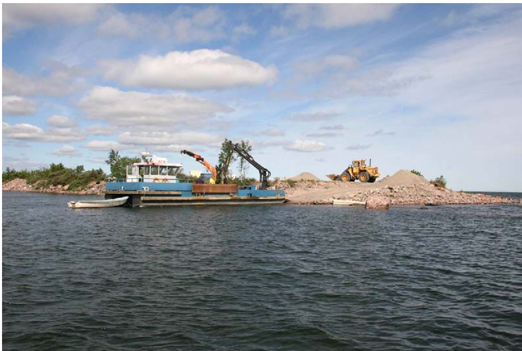
Figure 5-2. At the end of the pier at Asphällskulten a temporary slope was built in order to easily load or un-load the barge.
